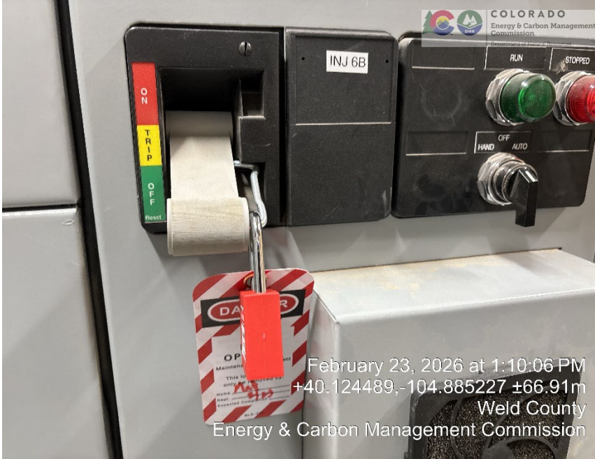
Electrical panel SI LOTO
