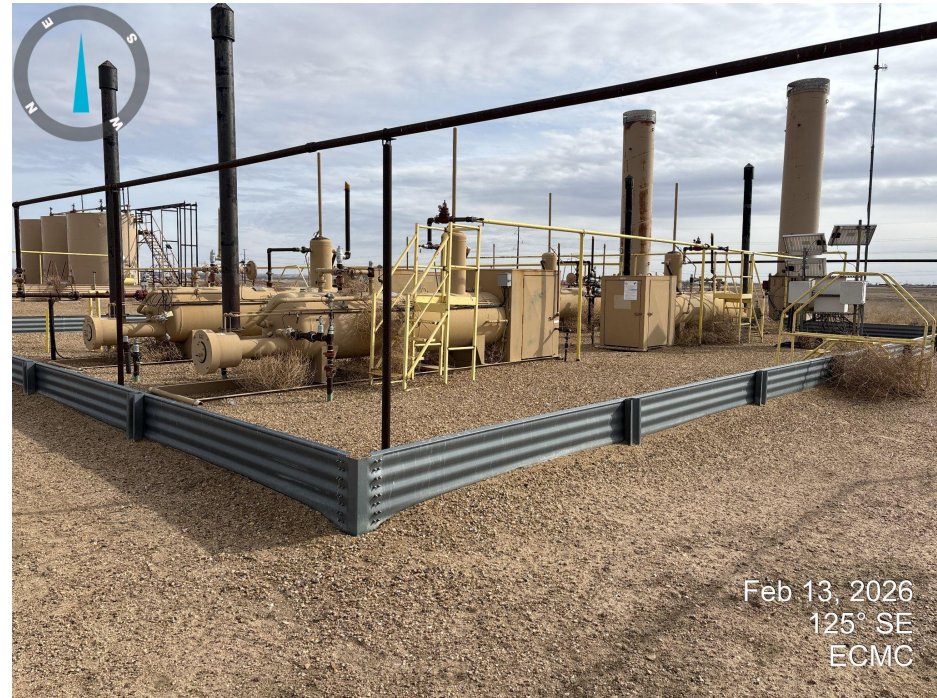
Photo 6. Separators at the tank battery have tumbleweed in contact with equipment.
