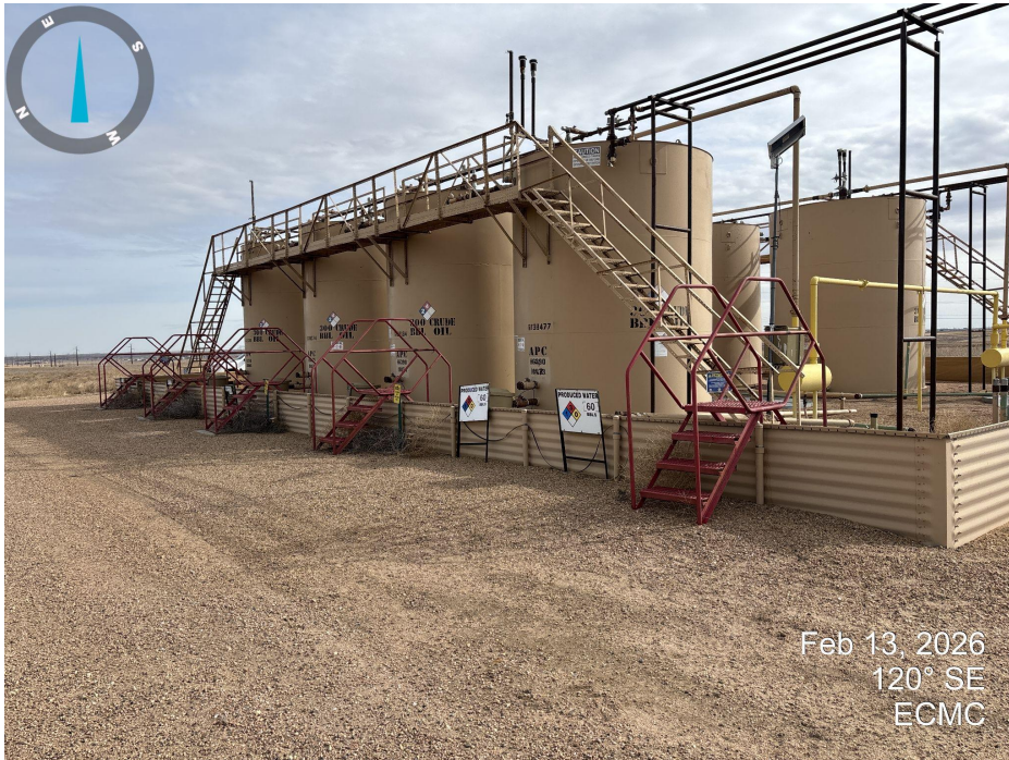
Photo 7. Storage tanks on the east side of the tank battery.
