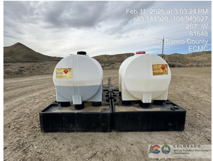
Photo # 2132 Chemical Labels starting to peel
