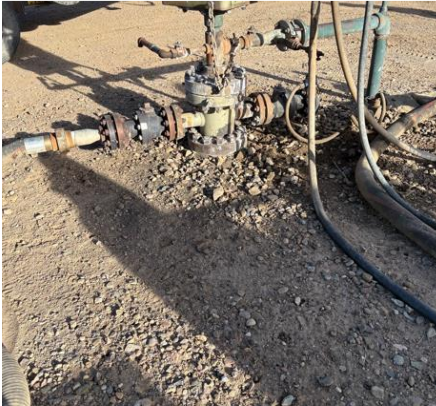
PHOTO 1: THE AREA OF IMPACTED SOIL AROUND THE WELLHEAD HAS BEEN REMOVED AND REPLACED WITH FRESH PAD MATERIAL. THE SELF INSPECTION PROCESS HAS BEEN REVIEWED AND THIS LOCATION WITH BE MONITORED FOR ANY FURTHER POTENTIAL COMPLIANCE ISSUES.
