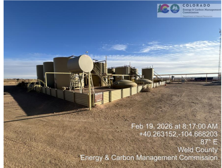
Photo 6 tank battery and equipment
