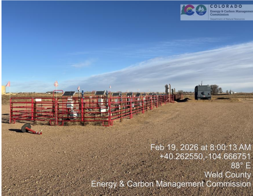
Photo 1 well heads and equipment
