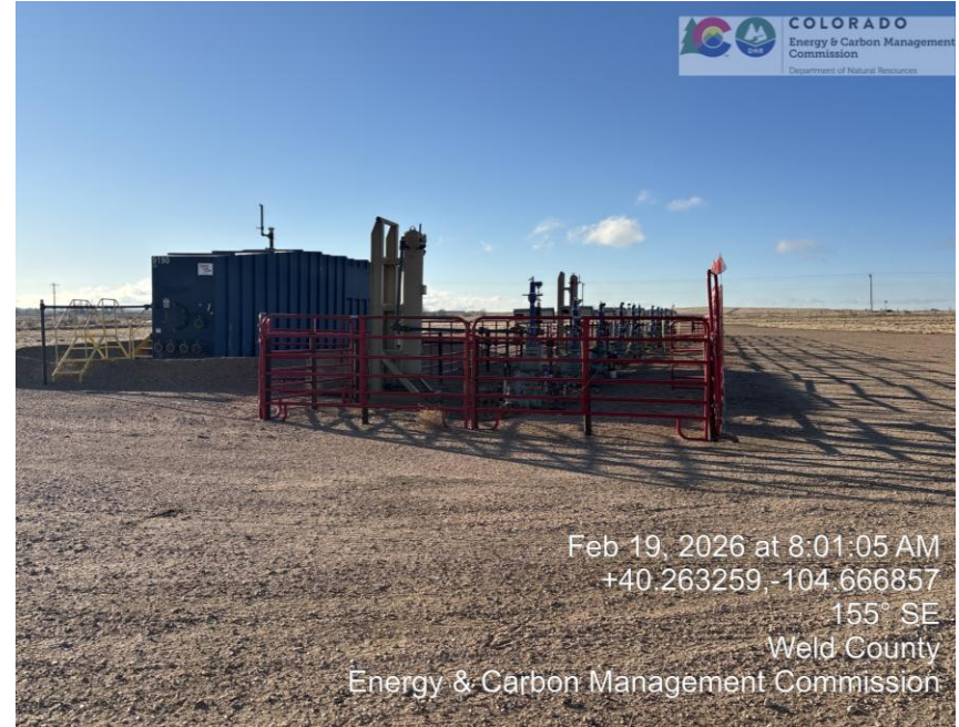
Photo 2 well heads and equipment
