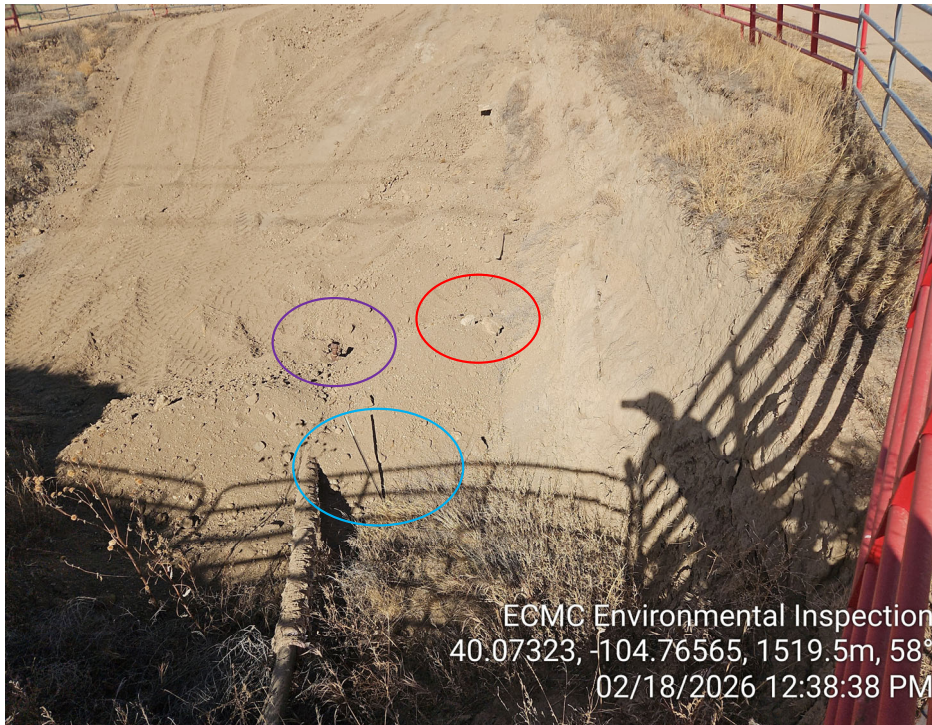
Photo 5 – Cement in backfill in open excavation (red). Uncapped pipe (purple) and t-post (blue) present in open excavation.
