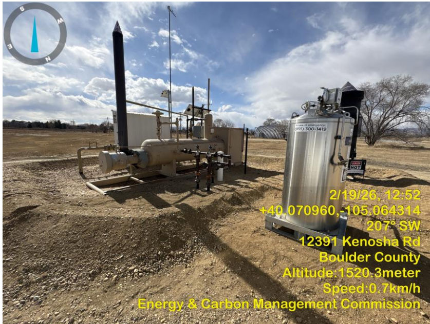
Photo 11 Horizontal Heated Separator & nitrogen tank.
