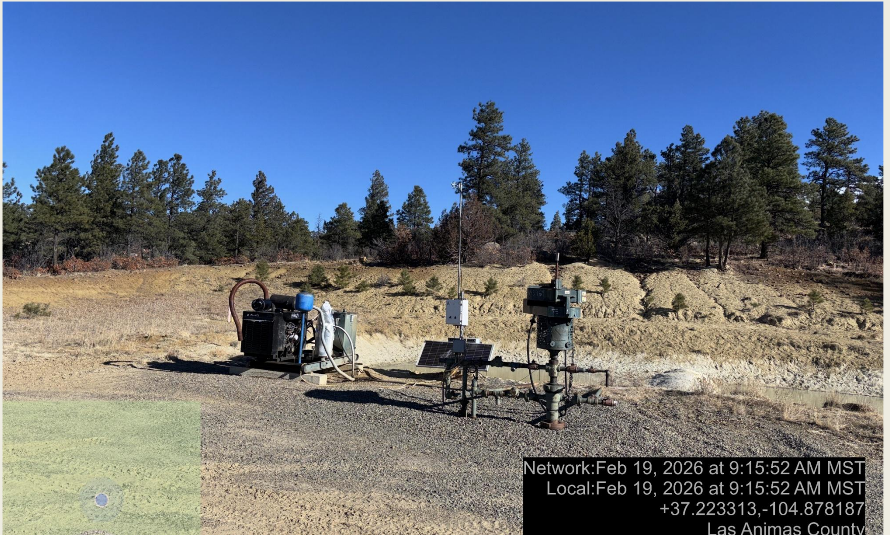
PHOTO 4: TR WELLHEAD AND EQUIPMENT.
