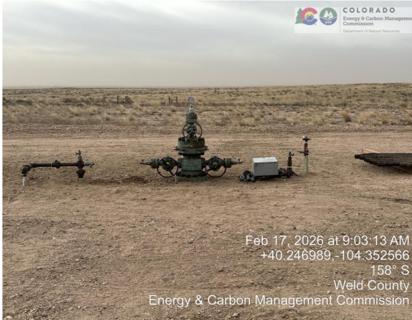
Photo 1 well head and equipment
