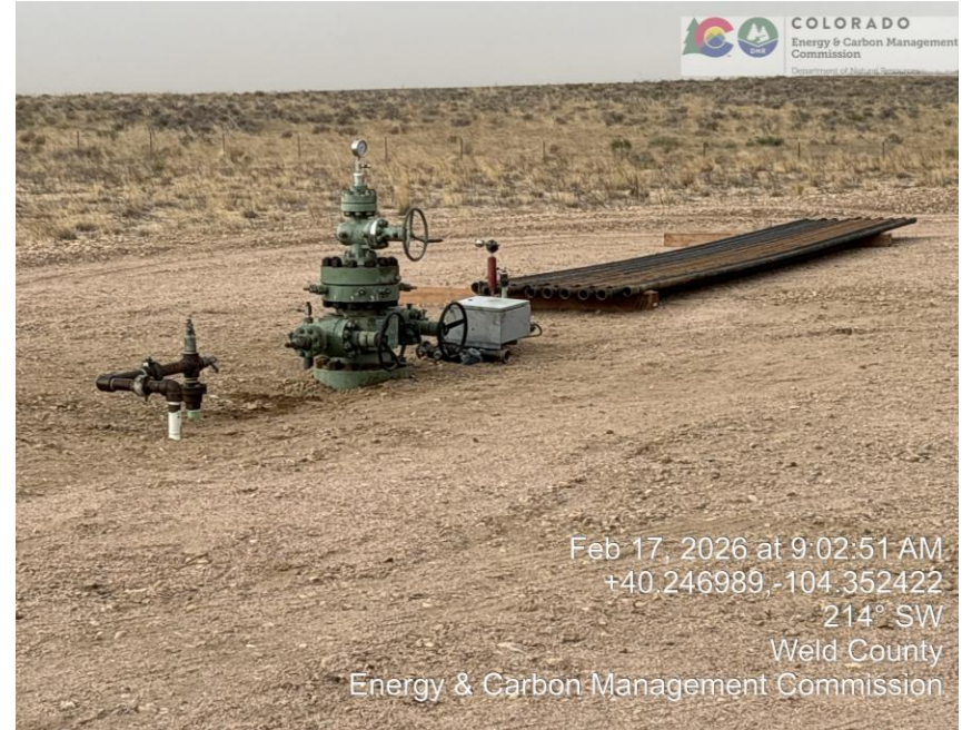
Photo 2 well head and equipment
