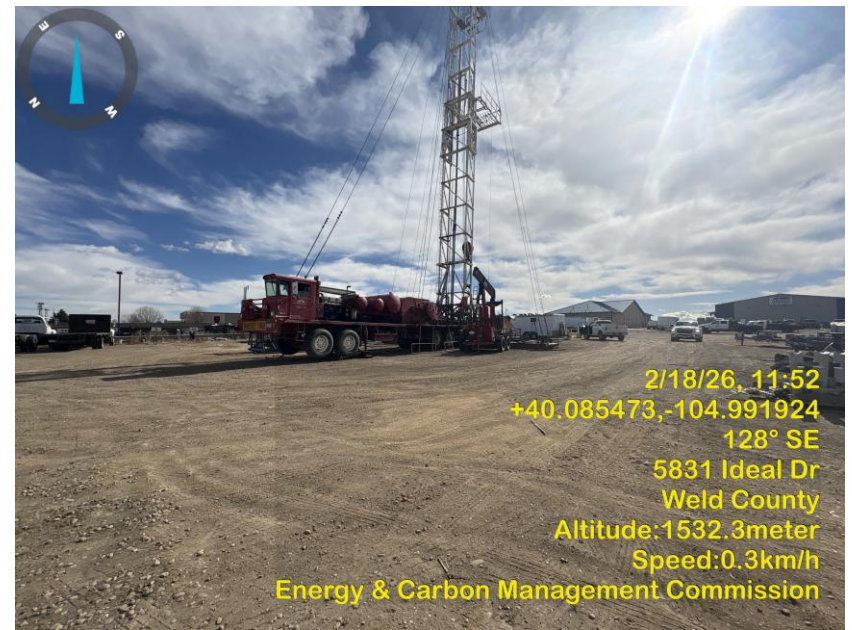
Photo 6 Accumulator trailer, Rig.
