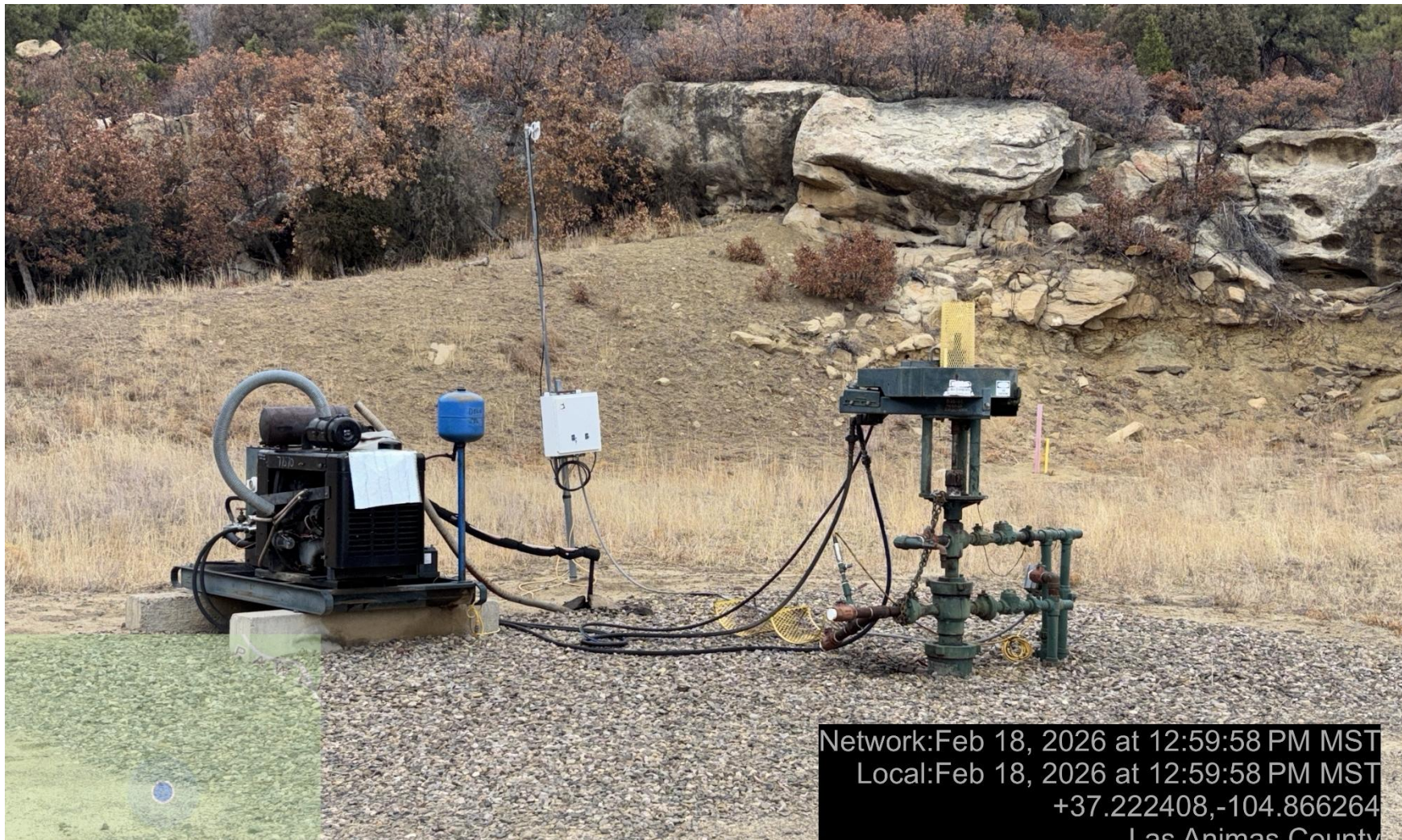
PHOTO 4: WELLHEAD AND EQUIPMENT.
