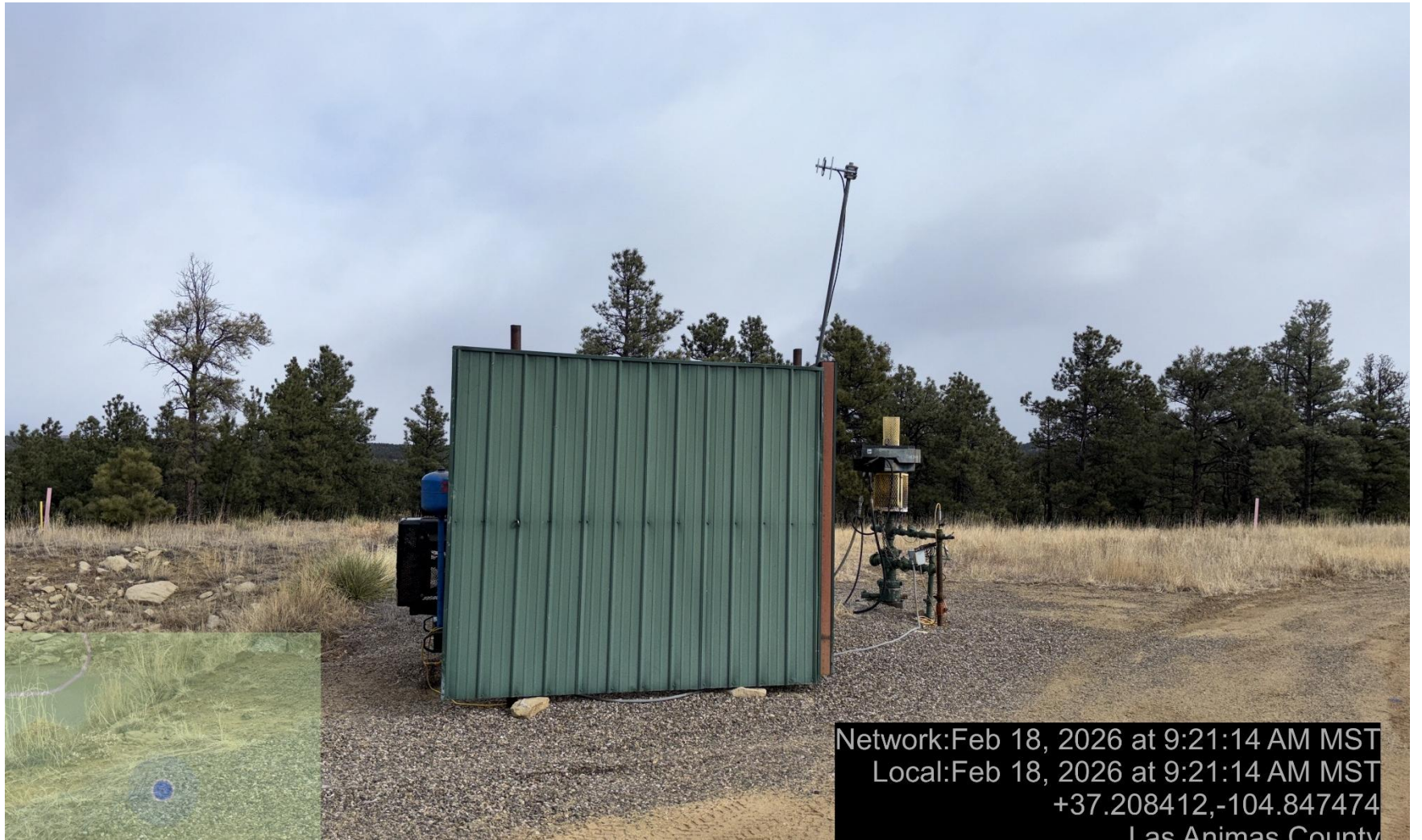
PHOTO 4: WELLHEAD AND EQUIPMENT.
