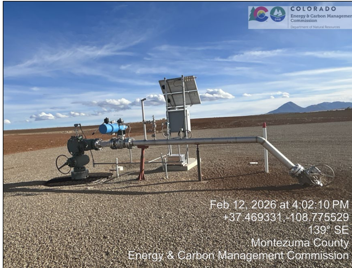
3. Wellhead, flow line, valves, and telemetry equipment.
