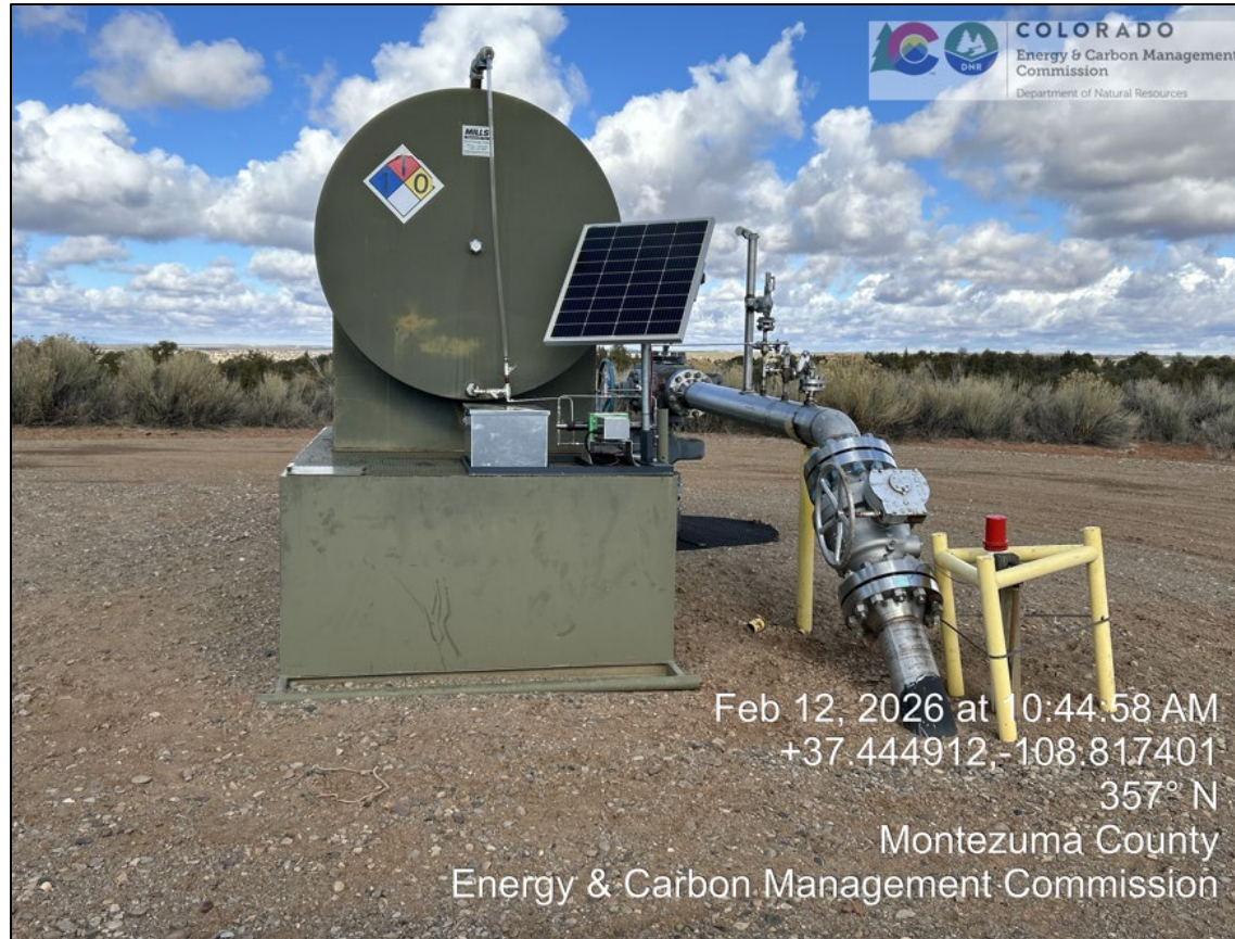
3. Tank and flow line. Hazcom placard visible.
