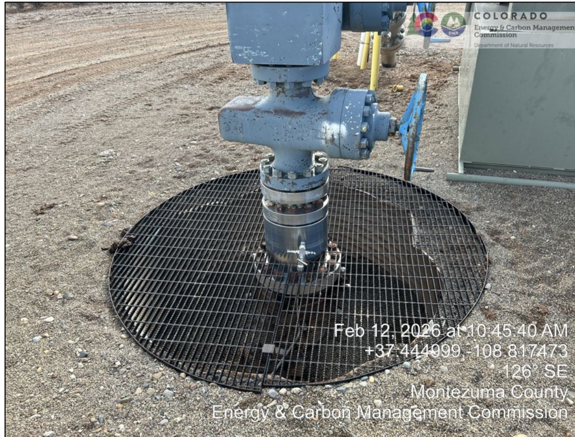
4. Well cellar, wellhead and bradenhead.
