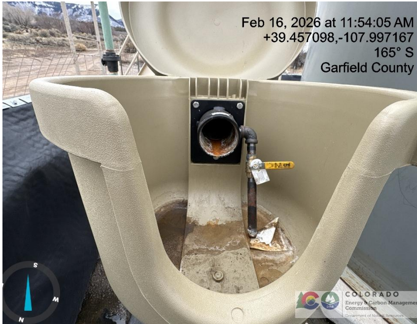
Photo # 9083 Open ended load line
