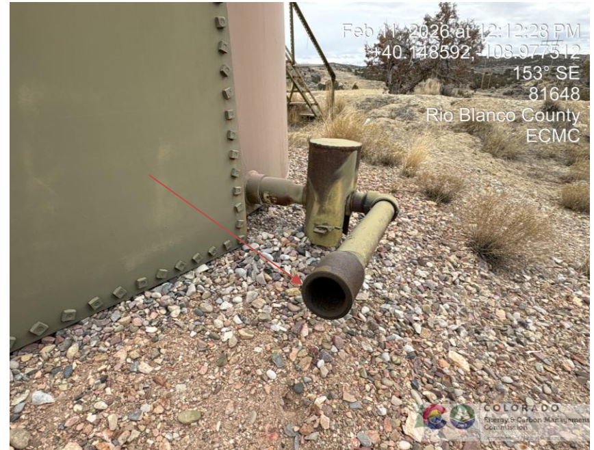
Photo # 2044 Open ended load line
