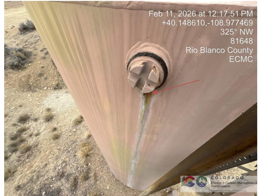
Photo # 2053 Production tank lacks integrity
