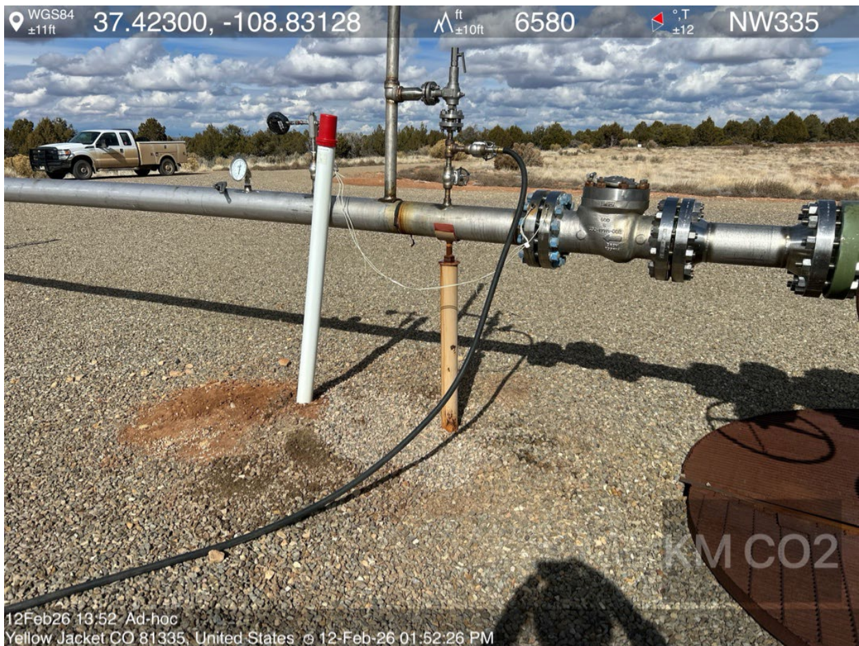
Photo #4. View of the GP-25 flowline and relief valve piping, with impacted soils removed.
