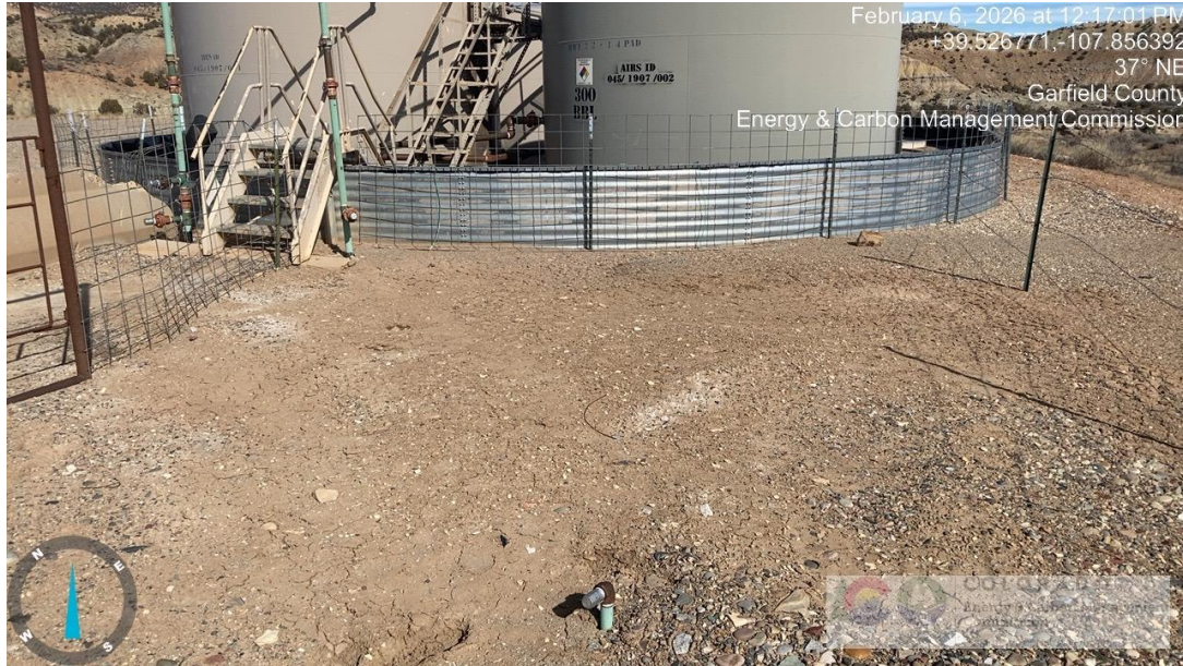
1" unused riser missing OOSLAT tag
