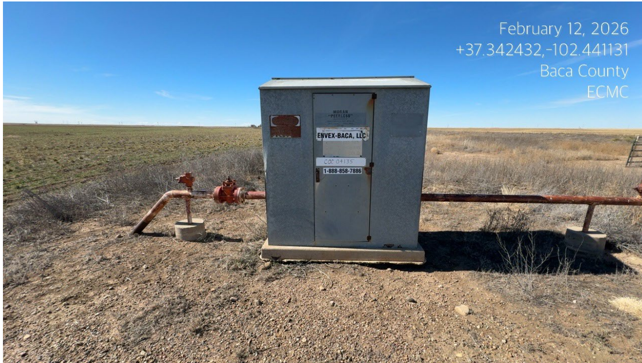
Photo 5. Sign post at the meter shed does not contain the required signage information.
