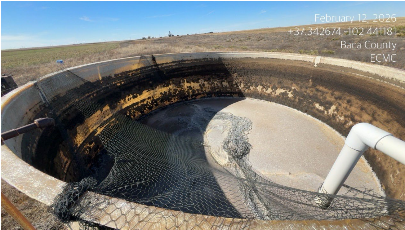
Photo 2. The netting on the open top tank is in disrepair.
