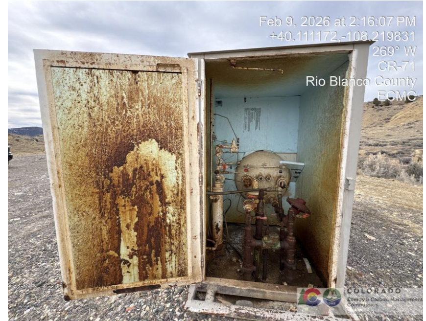
Photo # 1949 Staining at heater treater
