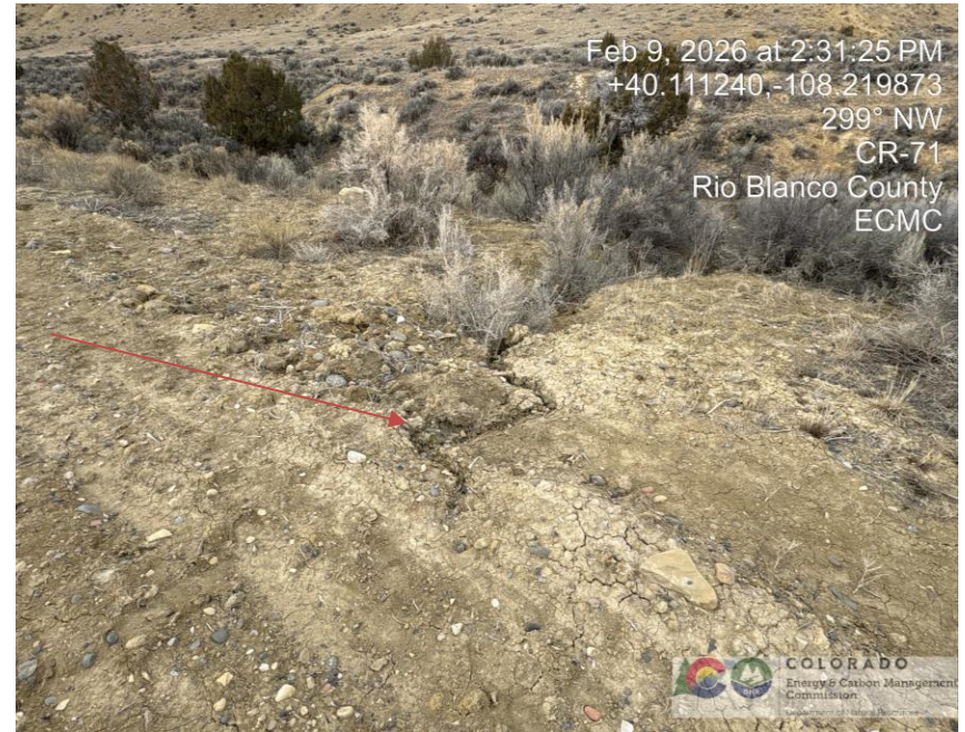
Photo # 1978 Failure to minimize erosion & transport of sediment off location/insufficient BMP's
