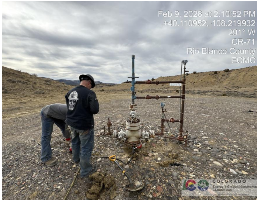
Photo # 1937 Wellhead seal test using Additel681AEx pressure gauge
