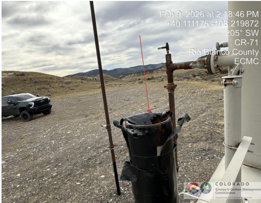
Photo # 1958 PRV vent line does not comply with CECMC pressure safety device rules
