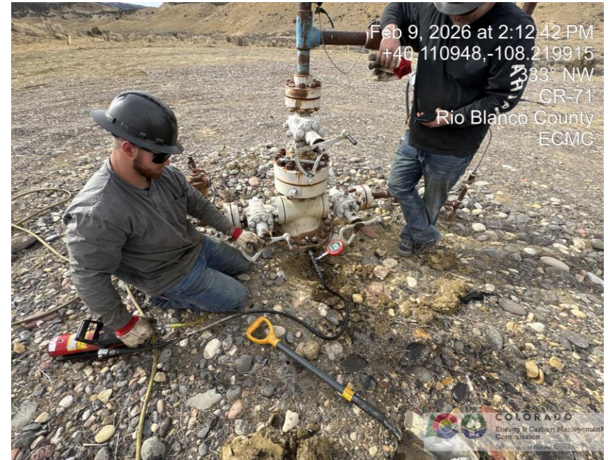
Photo # 1941 Wellhead seal test using Additel681AEx pressure gauge
