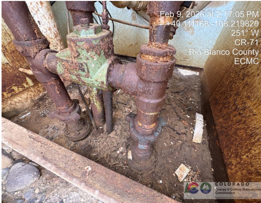
Photo # 1953 Staining at heater treater
