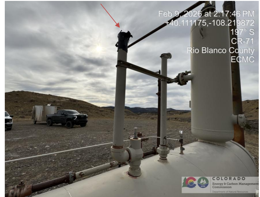
Photo # 1955 PRV vent line does not comply with CECMC pressure safety device rules
