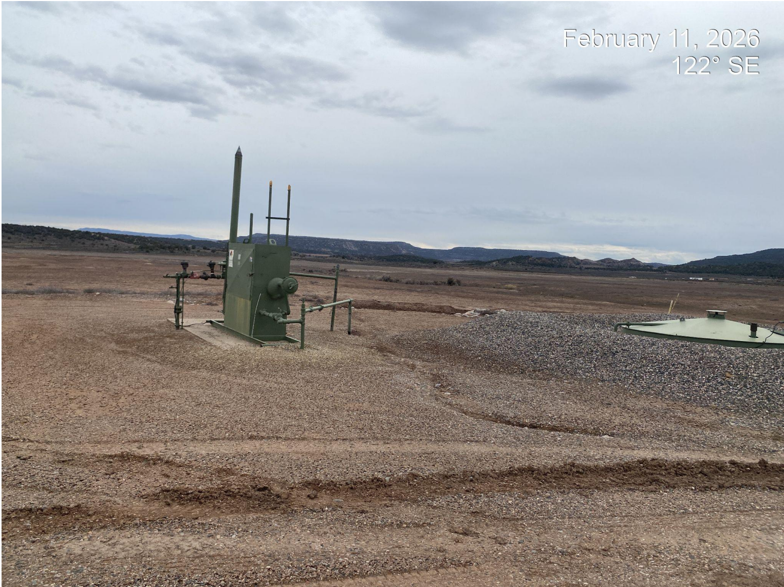
Photo 6. Erosion forming on the active pad.
