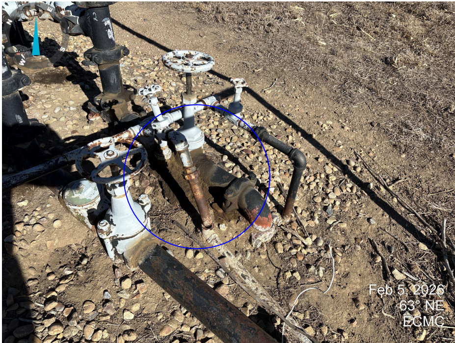
Photo 3. Photo taken at the south side of equipment. Stained soil/ oily buildup around joint (blue circle).
