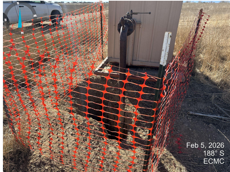
Photo 2. An excavation was present on the north side of the meter shed. A flowline was exposed below ground. Excavation was fenced. Several flags and markers were present around the location at appear to mark flowlines.
