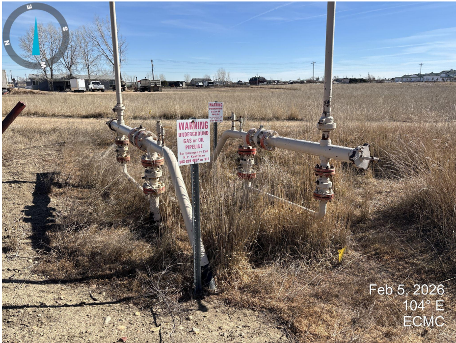
Photo 5. Flowline risers at the tank battery.
