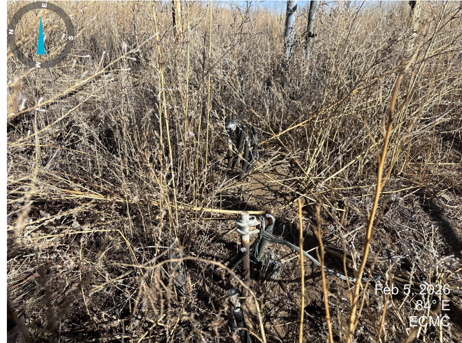
Photo 6. Photo taken in side the metal fence near the electric box. Cut off and exposed wires are present sticking out of the ground.
