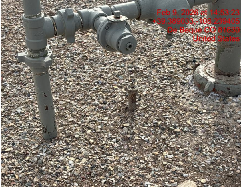
Open-Ended Line at Wellhead – Photo #02700
