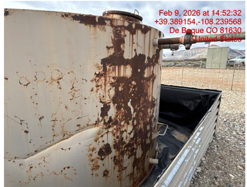
Corrosion on AST – Photo #02698
