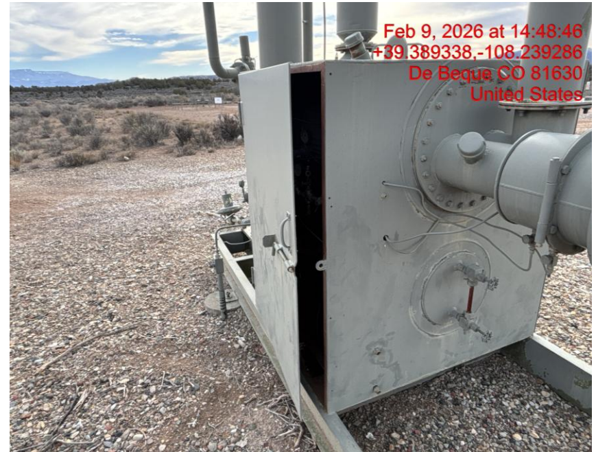
Unsecured Hatch/Wildlife Entry Hazard – Photo #02690
