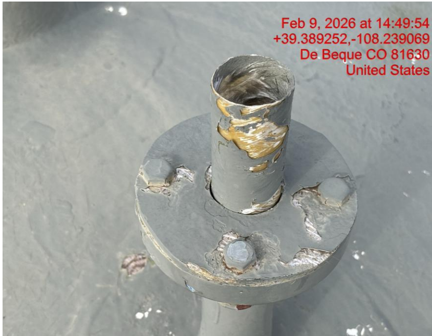
Open-Ended Vent on PBV – Photo #02693
