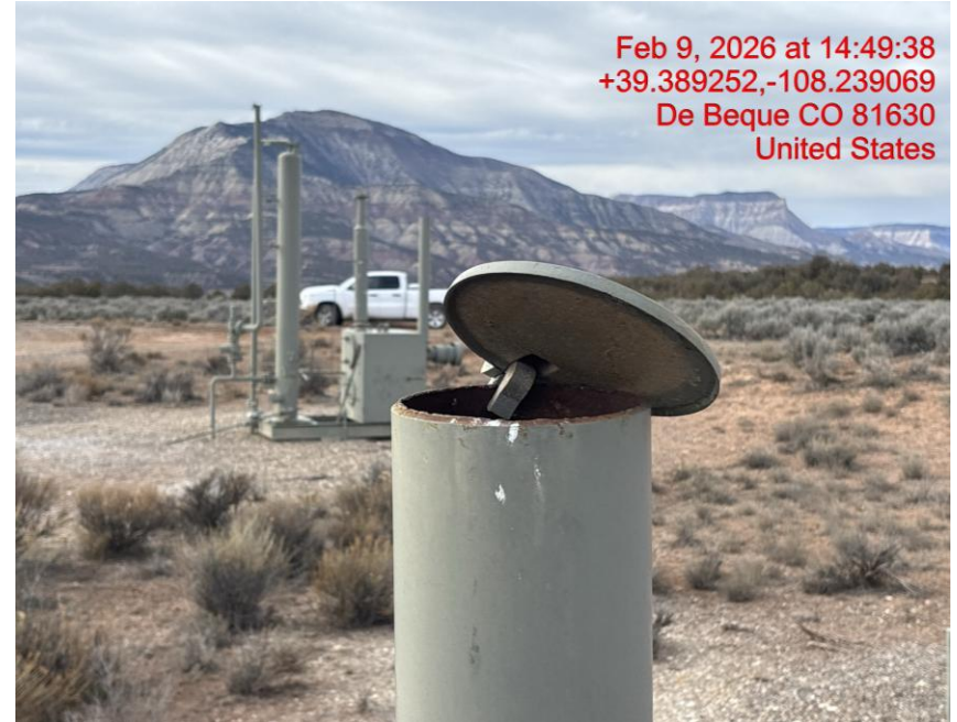
Open-Ended Vent on PBV – Photo #02692
