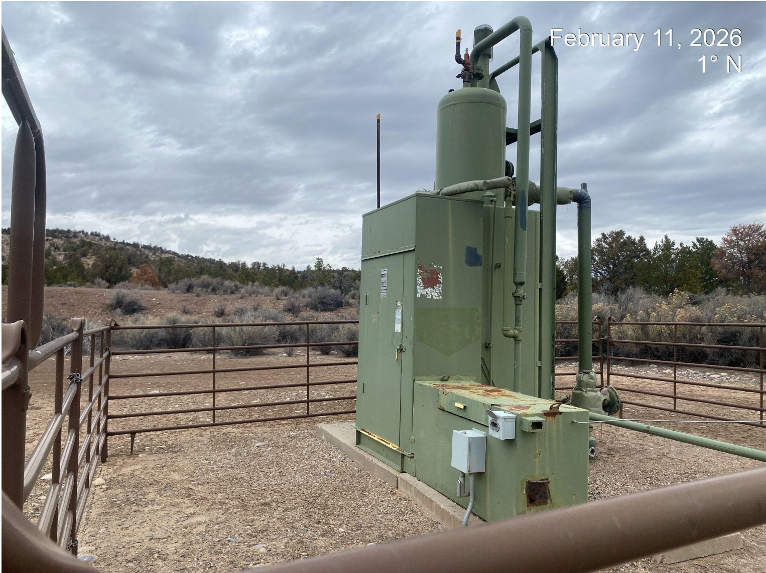
Photo 3. Label on separator equipment has deteriorated and is no longer legible.
