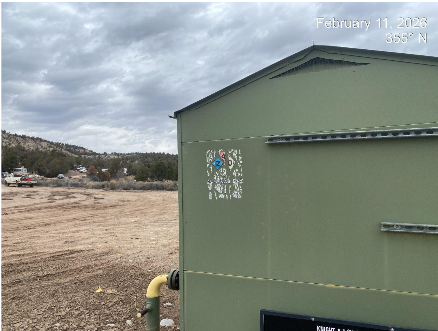
Photo 3. Label on meter shed has deteriorated and is no longer legible.
