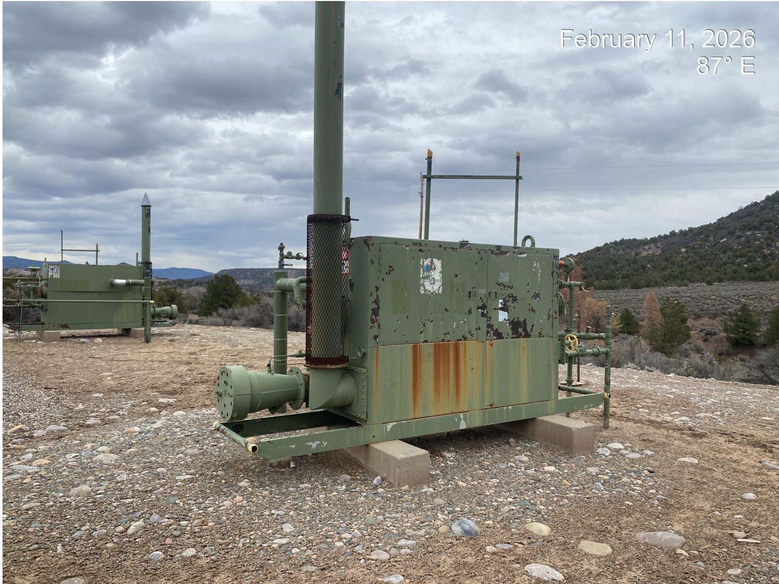
Photo 2. Separator labels have deteriorated and are no longer legible.
