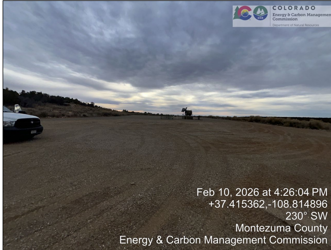
5. Well pad looking southwest from flow line assembly.
