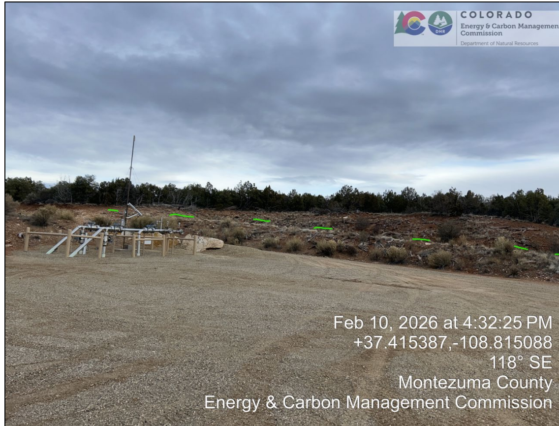
12. Run-on control ditch in cut slope on east side of pad indicated with dashed green line.
