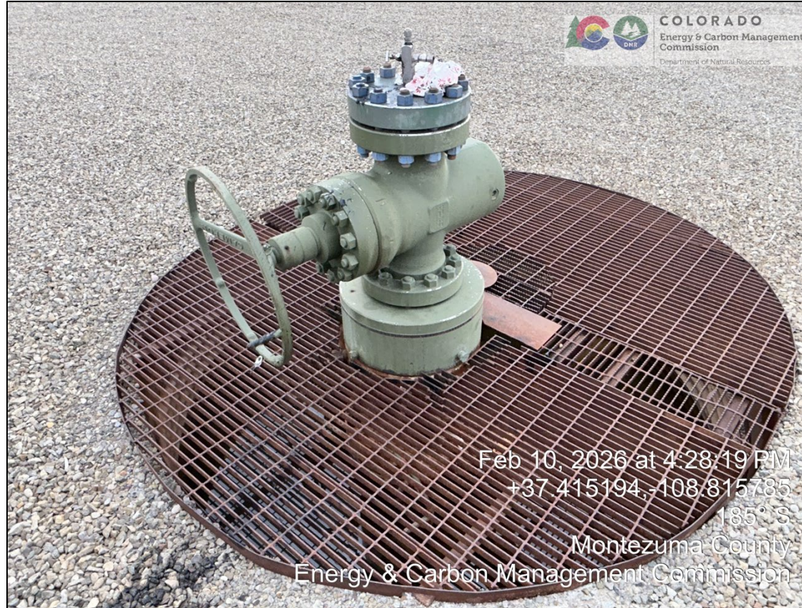
9. GP-21 wellhead and cellar. Bradenhead is accessible beneath grate. Note rag on top.
