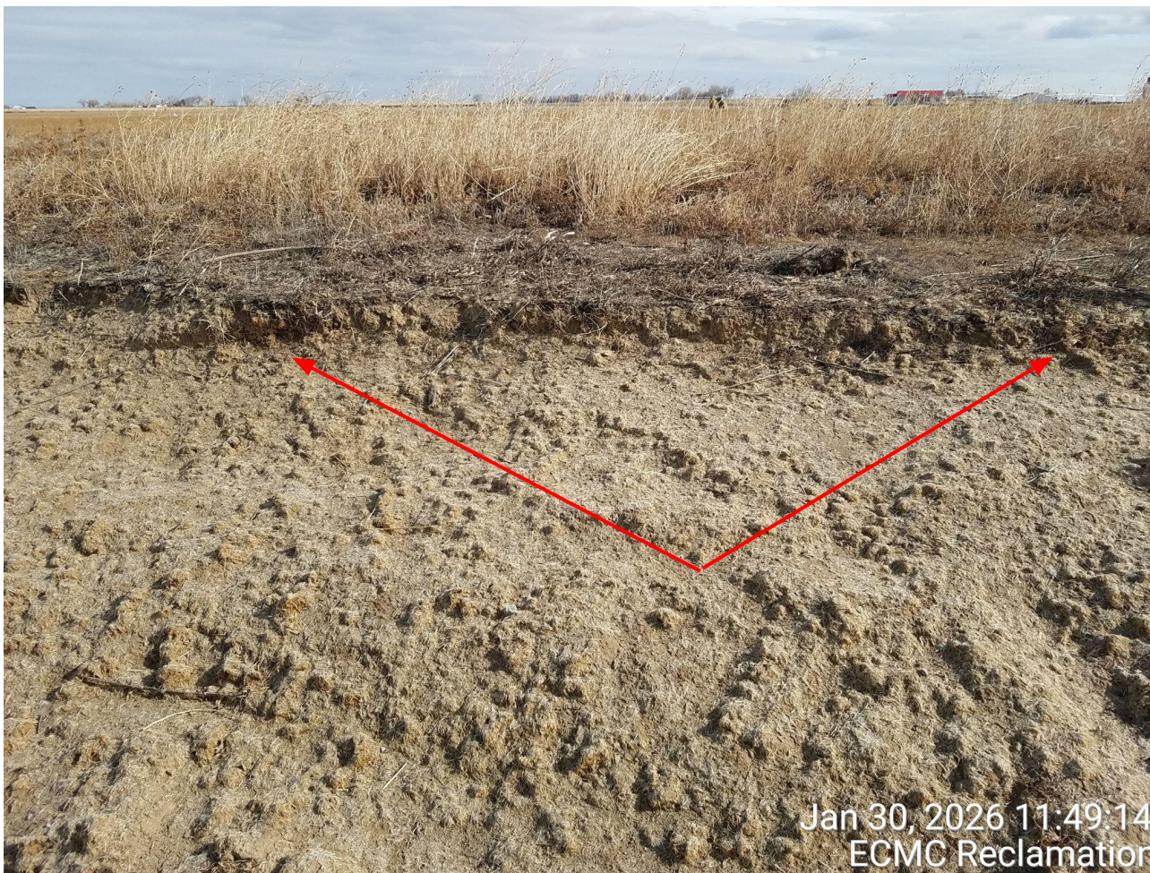
Photo 3. Photo taken from CR51 and the western portion of Parcel T089 near the surface owners driveway, facing East. Photo illustrates not all soil has been brought back to pre-disturbance conditions. Photo illustrates ~3-4 inches of soil material has not been brought back to the original contour.
