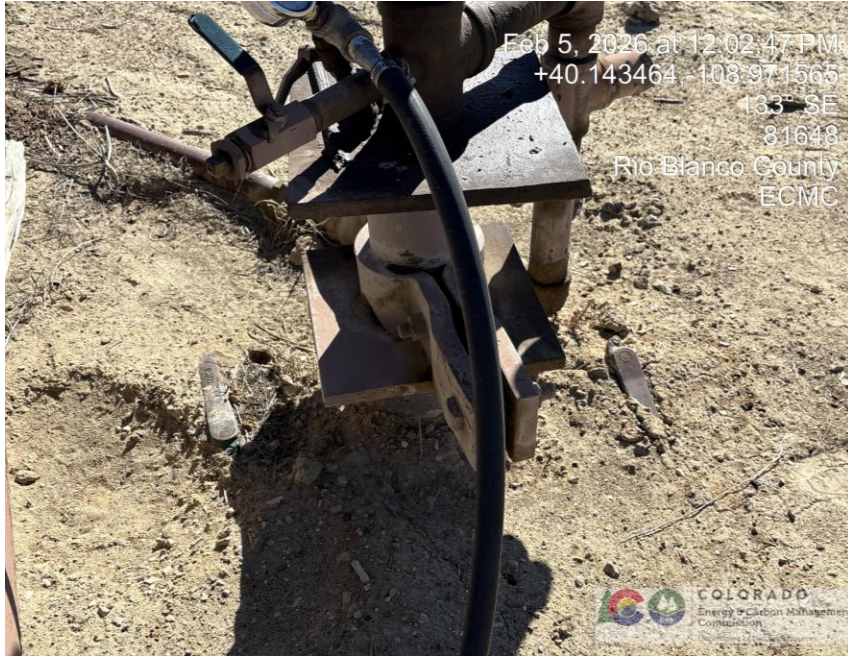
Photo # 1676 Bradenhead is inaccessible
