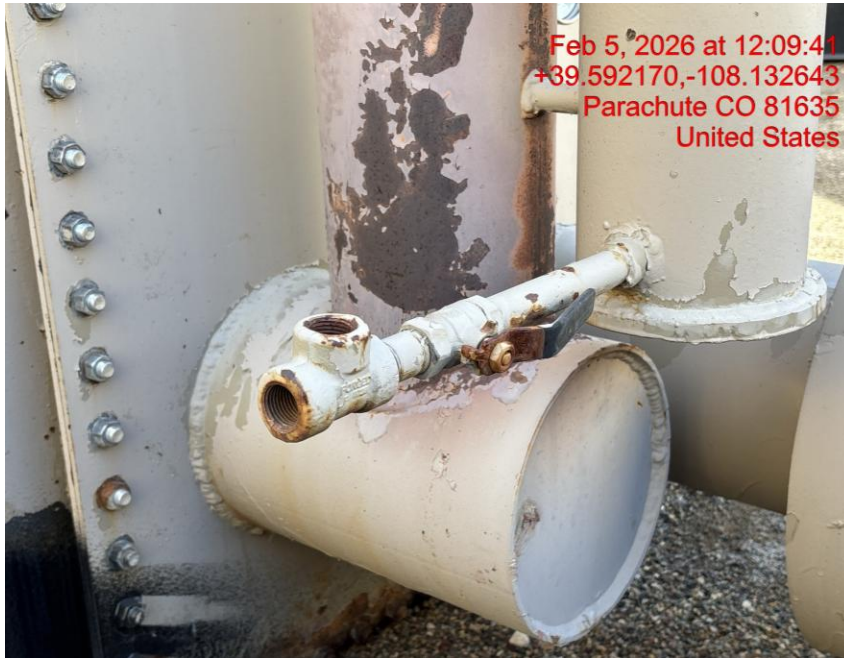
Open-Ended Line on Tank Burner Vessel – Photo #02651
