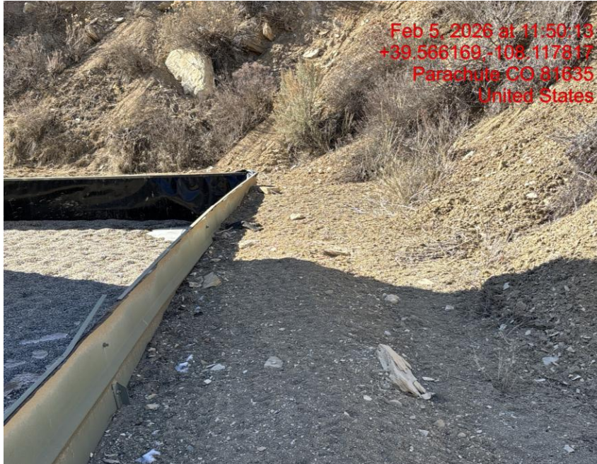
Cut Slope Erosion Encroaching into Secondary Containment – Photo #02638
