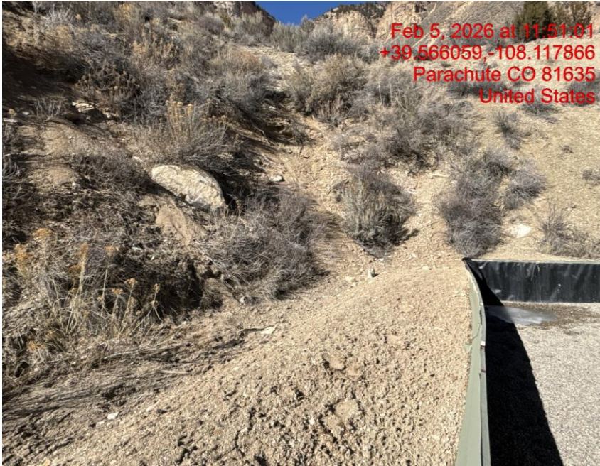
Cut Slope Erosion Encroaching into Secondary Containment – Photo #02642
