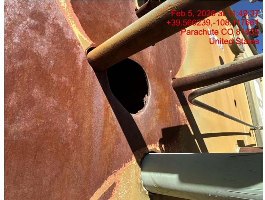
Wildlife Entry Hazard – Photo #02636
