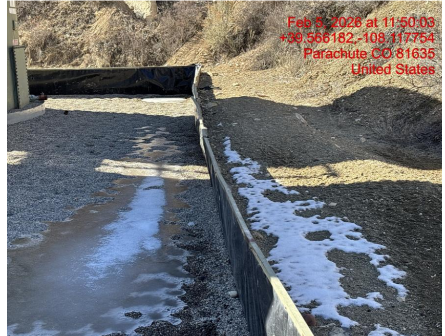
Cut Slope Erosion Encroaching into Secondary Containment – Photo #02637
