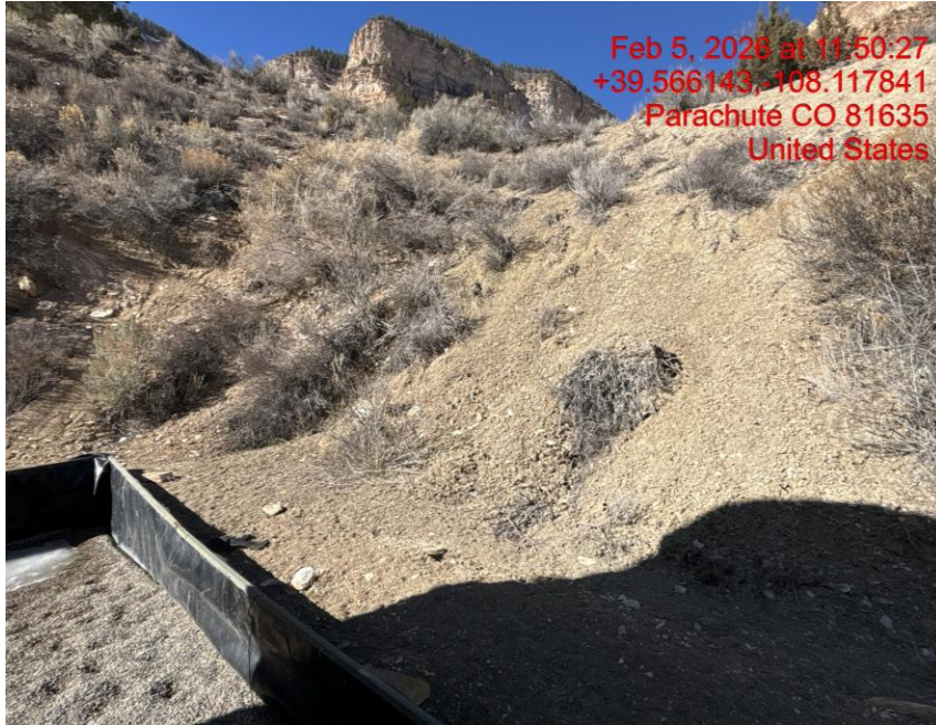
Insufficient Erosion Controls on Cut Slope – Photo #02639
