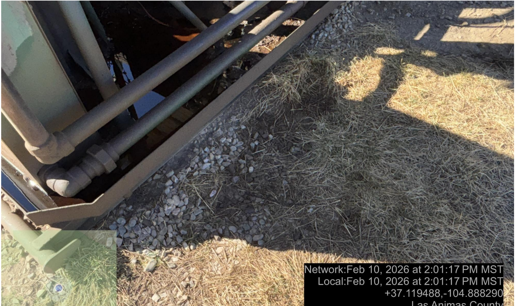
PHOTO 8: Area of impacted soil near compressor skid. Conduct maintenance on equipment, cleanup stained material and review self inspection processes. COMPLY WITH RULE 1002,.(2).D. ca date 2/23/2026.
