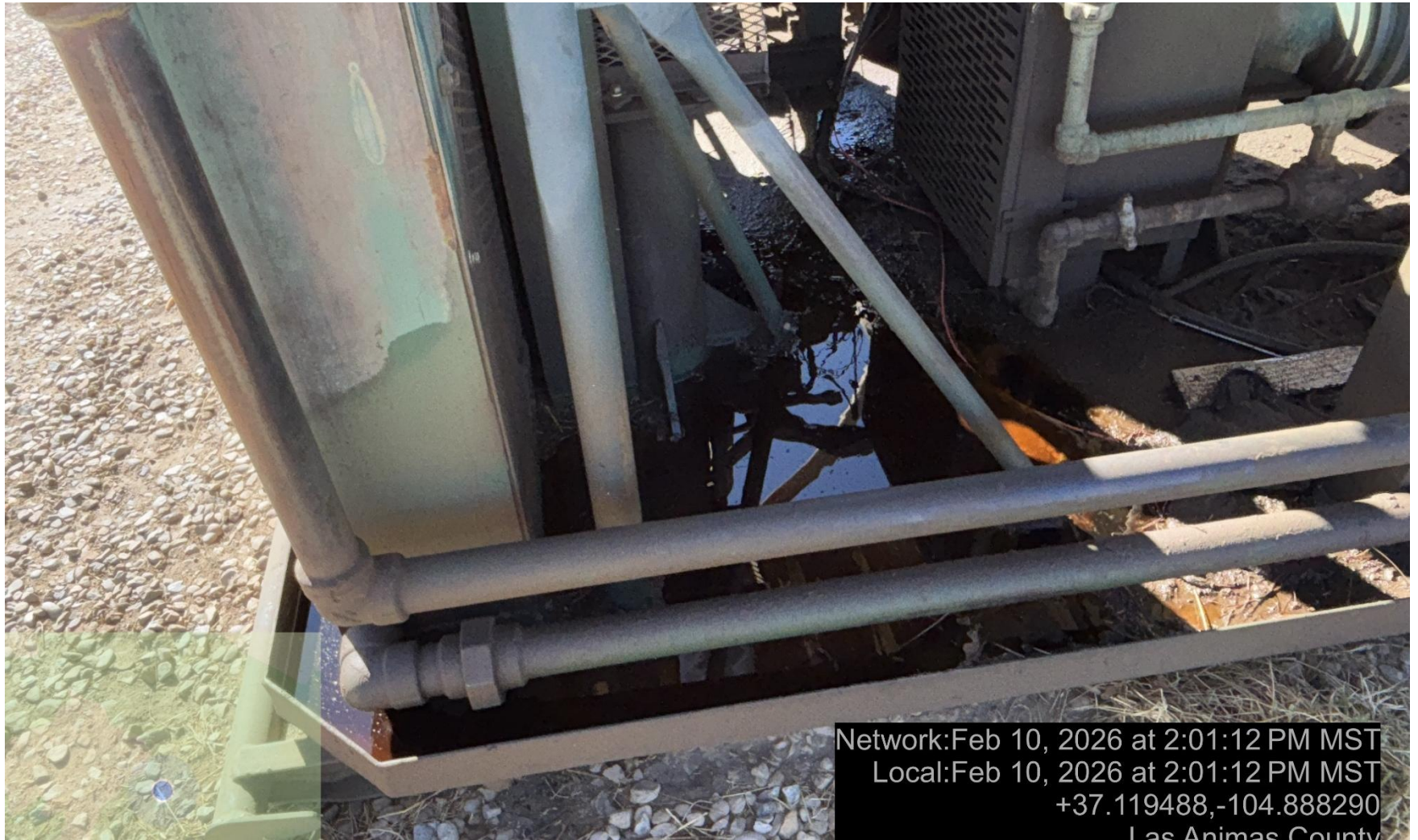
PHOTO 11: OILY WASTE IN COMPRESSOR SKID WITHOUT WILDLIFE PROTECTION SCREENS OR COVERS. DRAIN OILY WASTE REPAIR ALL LEAKS AND REMOVE IMPACTED SOIL PER RULE 1002..(2).D & 1002.f.(2)B, Comply with general provisions of the oil and gas act for wildlife protection AND SB-181. immediate action is required, ca date 2/11/2026.
