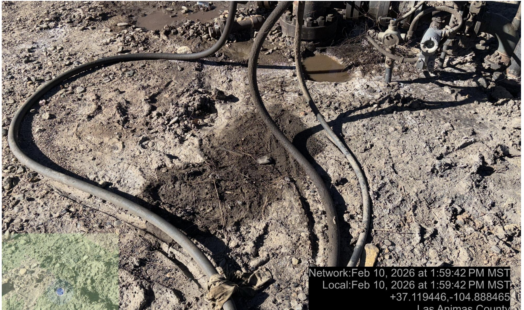
PHOTO 5: Area of impacted soil near wellhead appears to be from leaking hydraulic hose. Conduct maintenance on equipment, cleanup stained material and review self inspection processes. COMPLY WITH RULE 1002,(2).D. ca date 2/23/2026.
