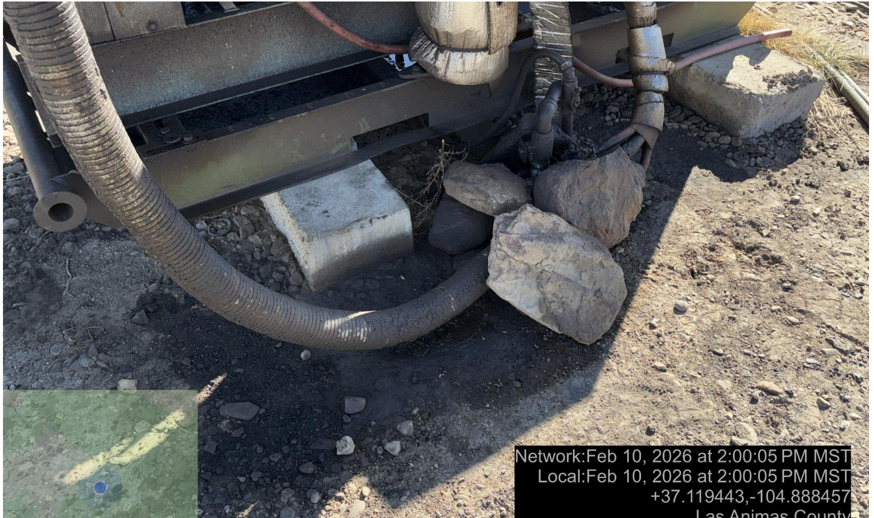
PHOTO 7: Area of impacted soil near prime mover engine skid. Conduct maintenance on equipment, cleanup stained material and review self inspection processes. COMPLY WITH RULE 1002,(2).D. ca date 2/23/2026.
