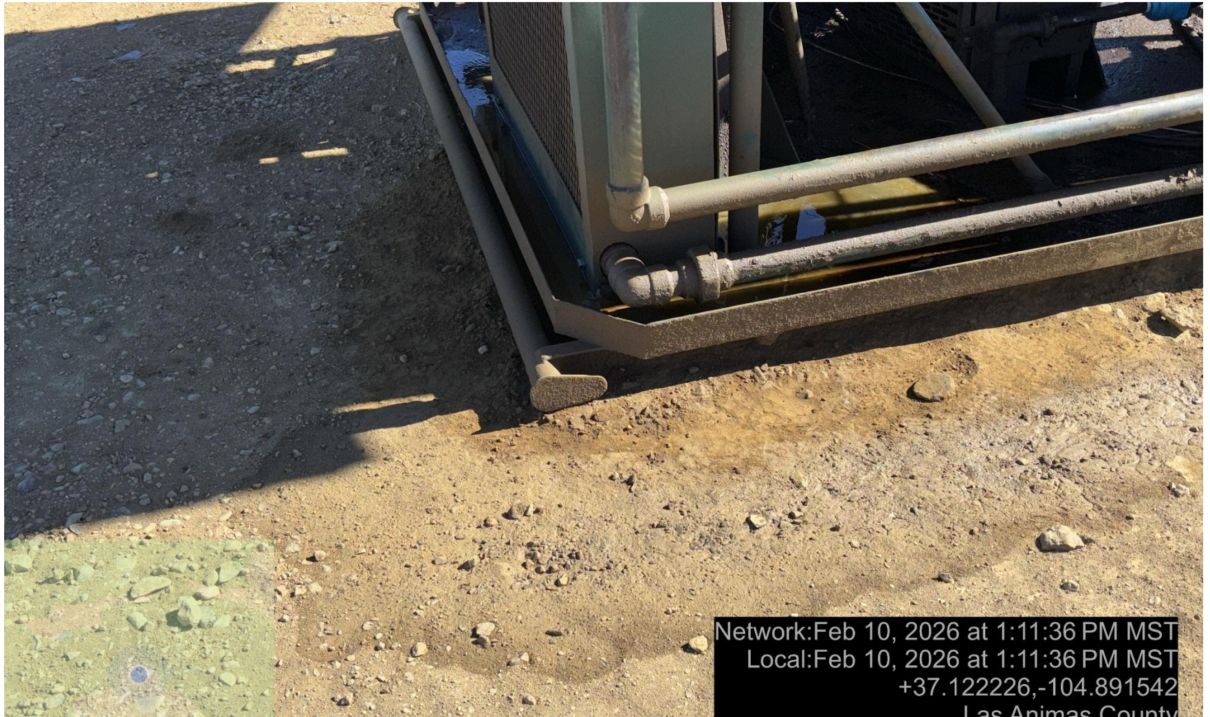
PHOTO 6: area of impacted soil near compressor skid. Conduct maintenance on equipment, cleanup stained material and review self inspection processes. COMPLY WITH RULE 1002,.(2).D. ca date 2/23/2026.
