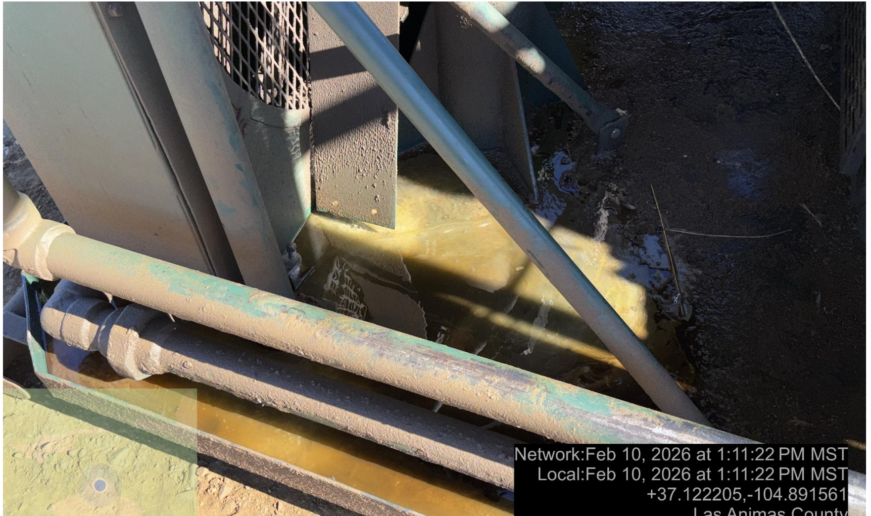
PHOTO 12: OILY WASTE IN COMPRESSOR SKID WITHOUT WILDLIFE PROTECTION SCREENS OR COVERS. DRAIN OILY WASTE REPAIR ALL LEAKS AND REMOVE IMPACTED SOIL PER RULE 1002..(2).D & 1002.f.(2)B, Comply with general provisions of the oil and gas act for wildlife protection AND SB-181. IMMEDIATE ACTION IS REQUIRED. CA DATE 2/11/2026.
