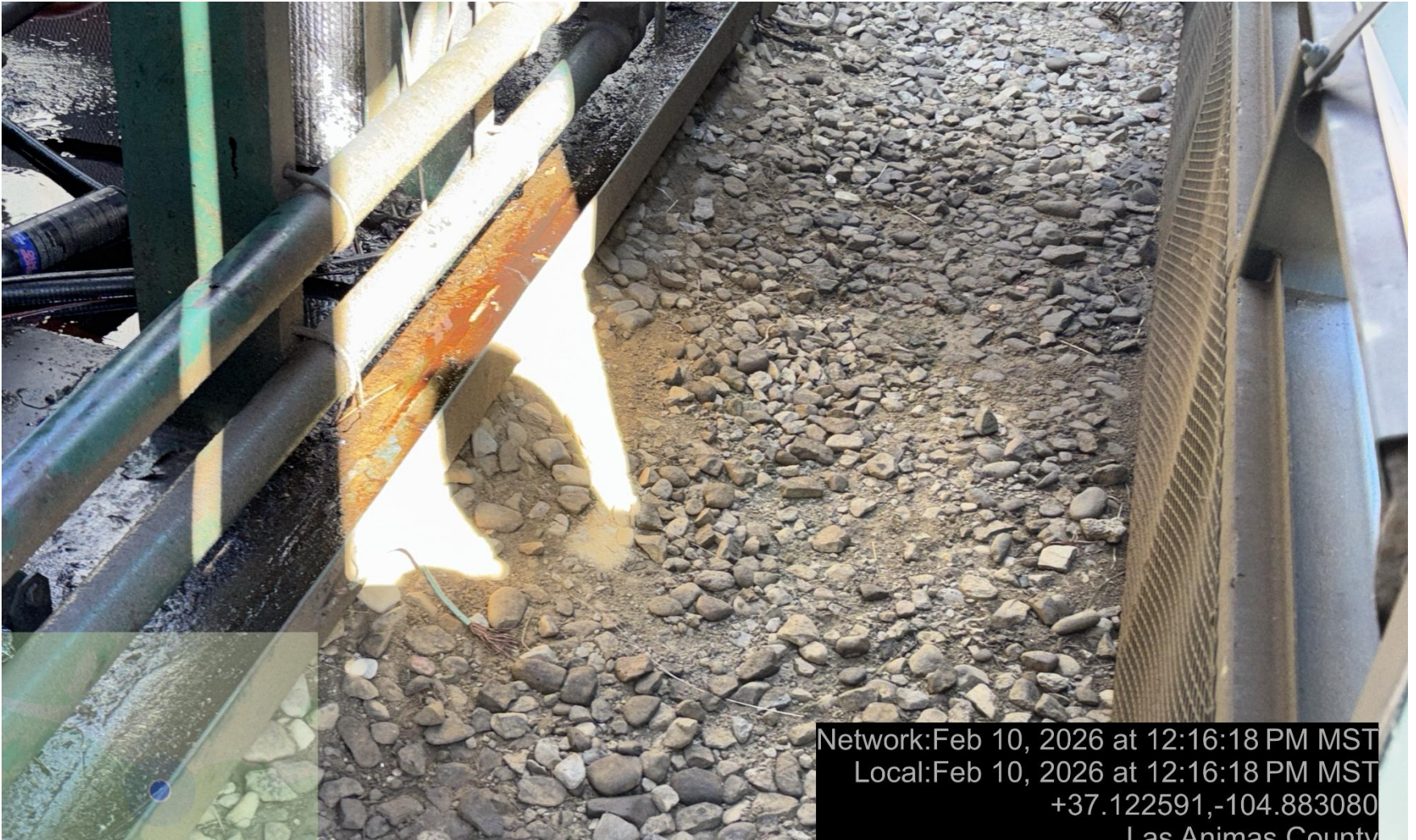
PHOTO 8: area of impacted soil near compressor appears to be from leaking equipment over an extended period of time. Conduct maintenance on equipment, cleanup stained material and review self inspection processes. COMPLY WITH RULE 1002,.(2).D. ca date 2/23/2026.
