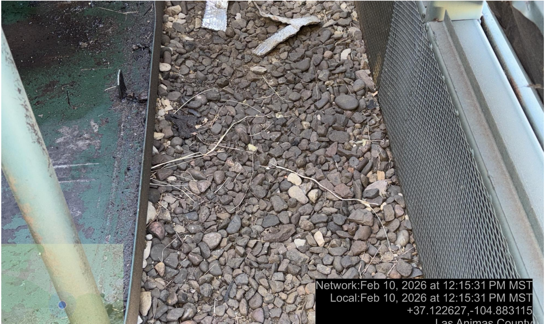
PHOTO 8: area of impacted soil near compressor appears to be from leaking equipment over an extended period of time. Conduct maintenance on equipment, cleanup stained material and review self inspection processes. COMPLY WITH RULE 102,.(2).D. ca date 2/23/2026.
