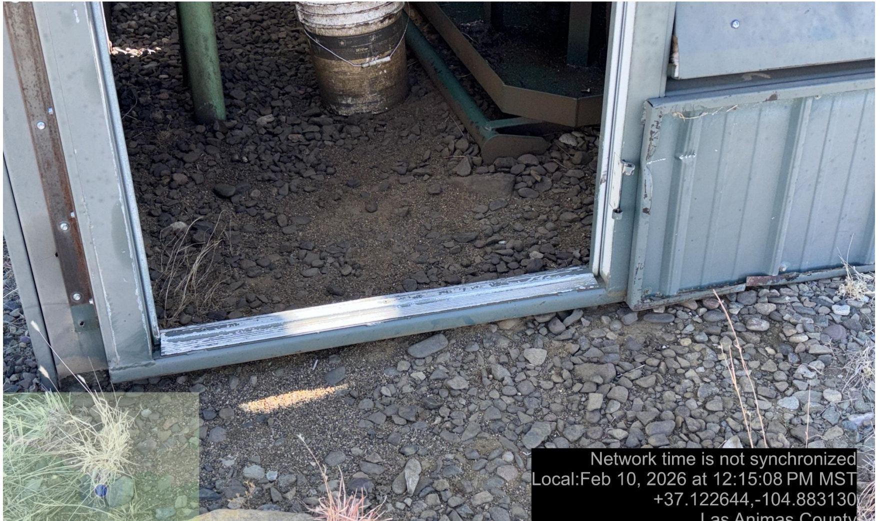
PHOTO 7: area of impacted soil near compressor appears to be from leaking equipment over an extended period of time. Conduct maintenance on equipment, cleanup stained material and review self inspection processes. COMPLY WITH RULE 1002,(2).D. ca date 2/23/2026.
