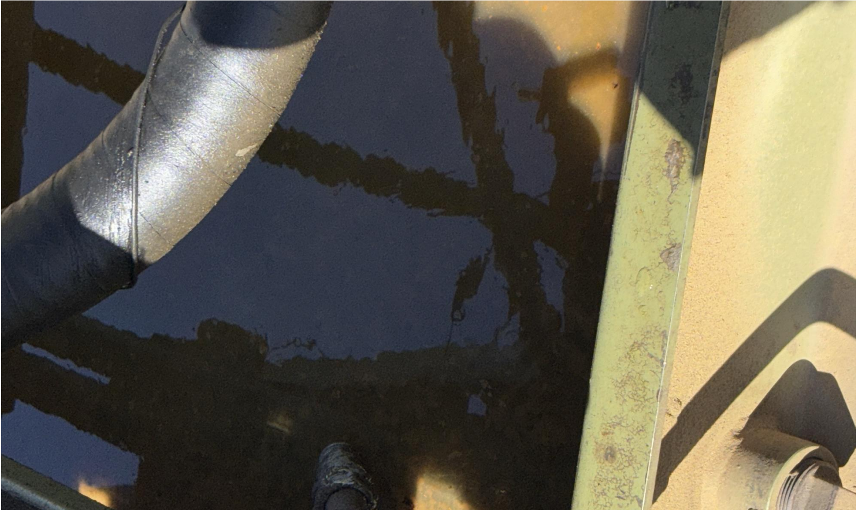
PHOTO 11: oily waste in prime mover engine skid without wildlife protections in place. DRAIN OILY WASTE REPAIR ALL LEAKS AND REMOVE IMPACTED SOIL PER RULE 1002..(2).D & 1002.f.(2)B, Comply with general provisions of the oil and gas act for wildlife protection AND SB-181. this equipment is leaking so bad in should be taken out of service until leaks are repaired. Ca date 2/11/2026.
