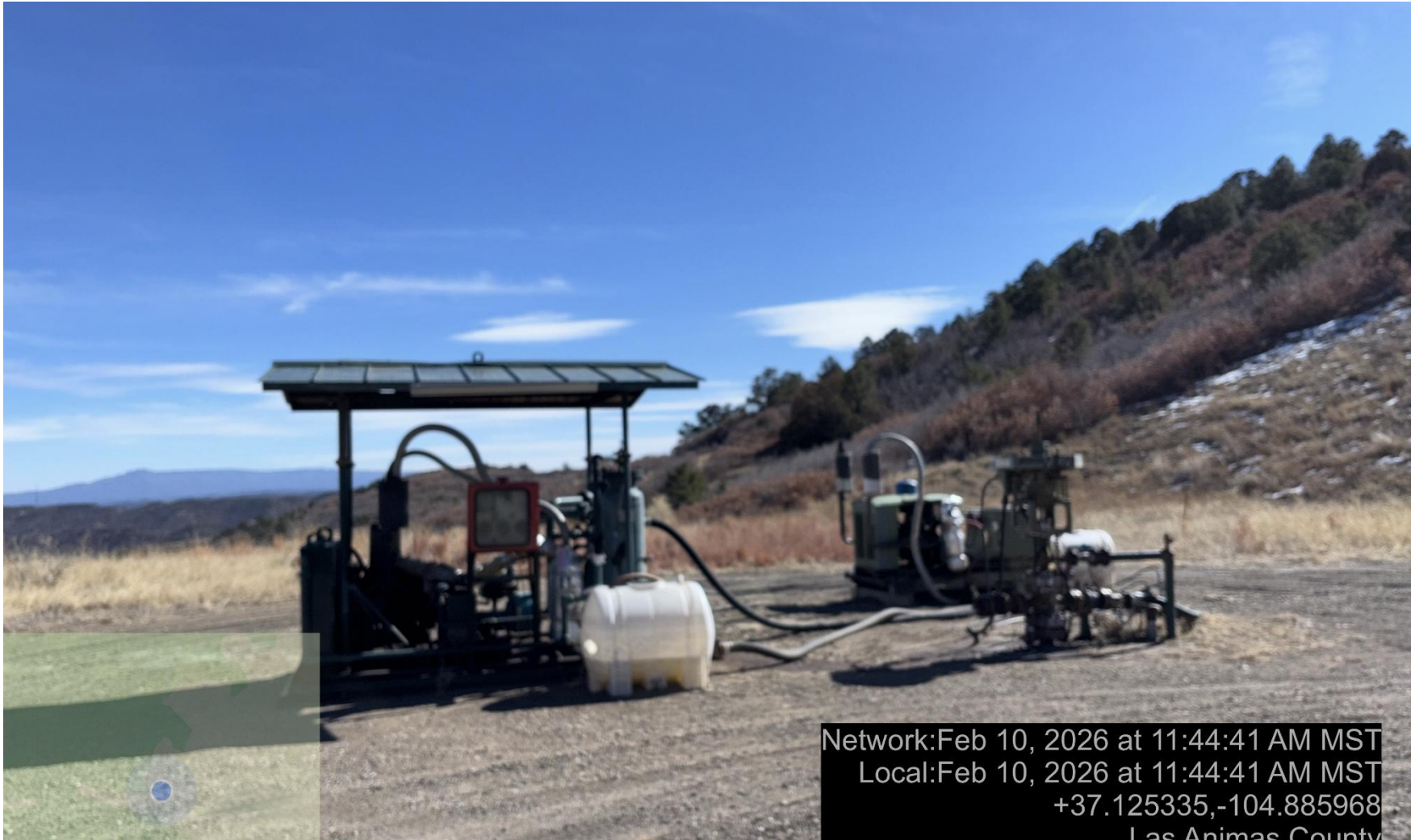
PHOTO 4: Vacuum pump observed on well without ECMC approval. Provide ECMC with documentation showing approval of use of vacuum pump. Ca date 2-27-2026.
