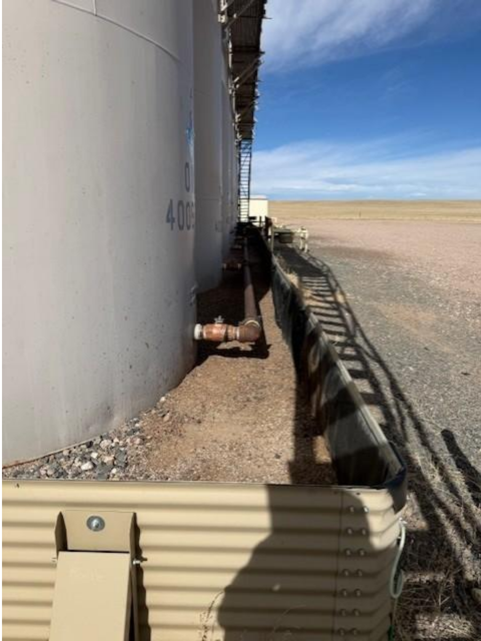
Photo #9 Motu East 2821 - 8CH Tank Battery
