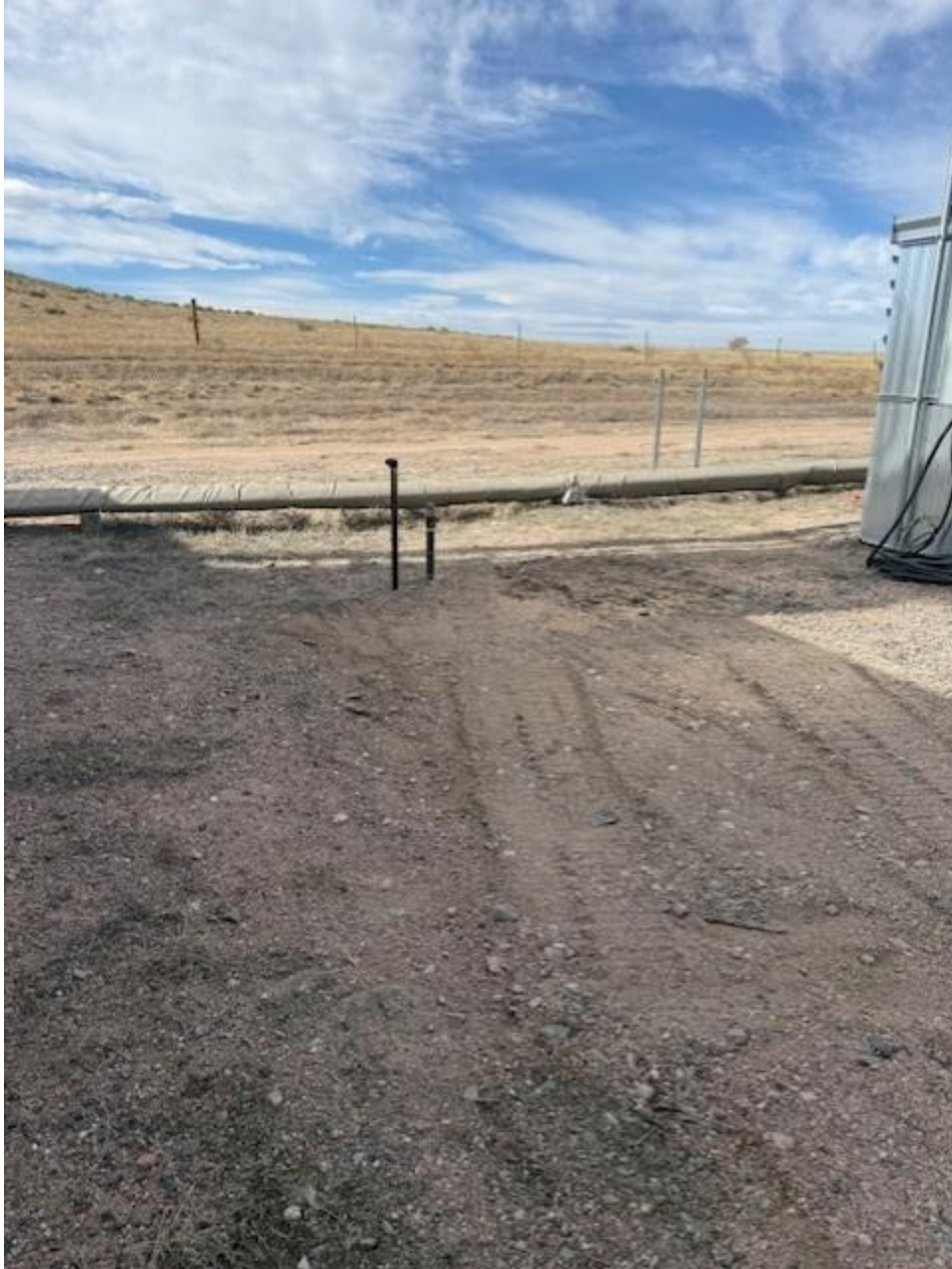
Photo #5 Motu East 28-21-16-1CH Wellsite - Stained soil, trash
