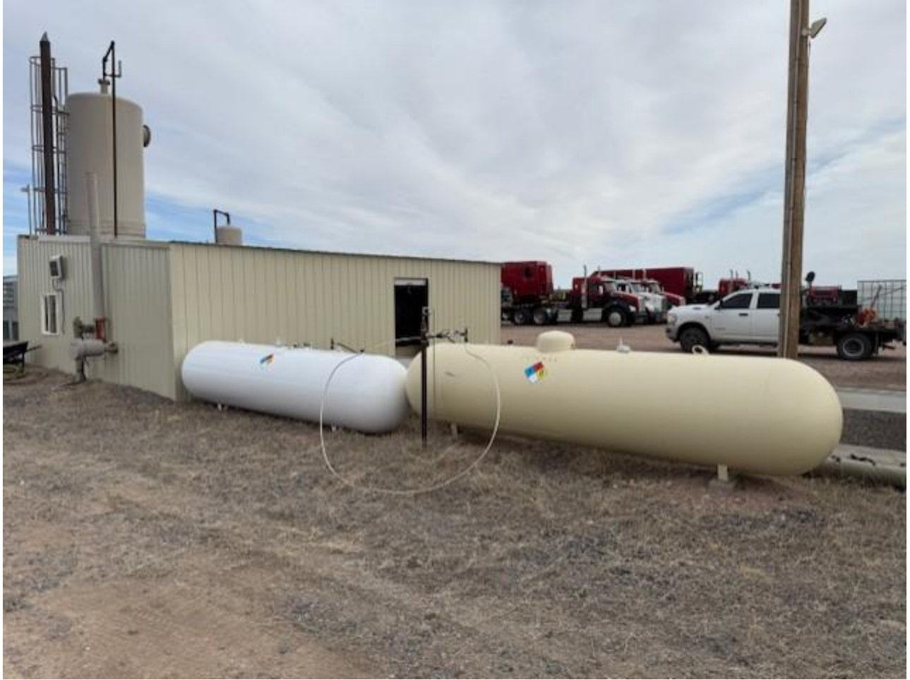
Photo #3 Motu East 28-21-16-1CH Pump House with outdoor tanks
