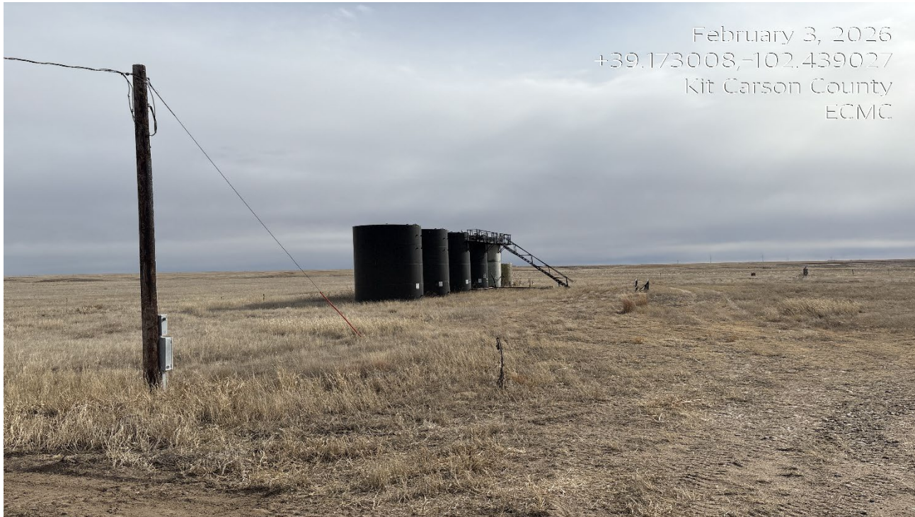
Photo 1. Facing southeast toward the location. The electric utility needs to be removed. All tanks equipment must be removed..
