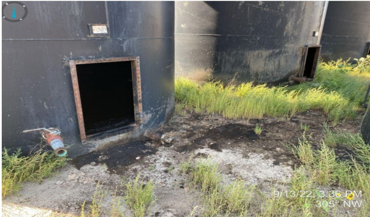
Photo 4. Photo taken during previous inspection shows E&P waste spill out onto the ground..
