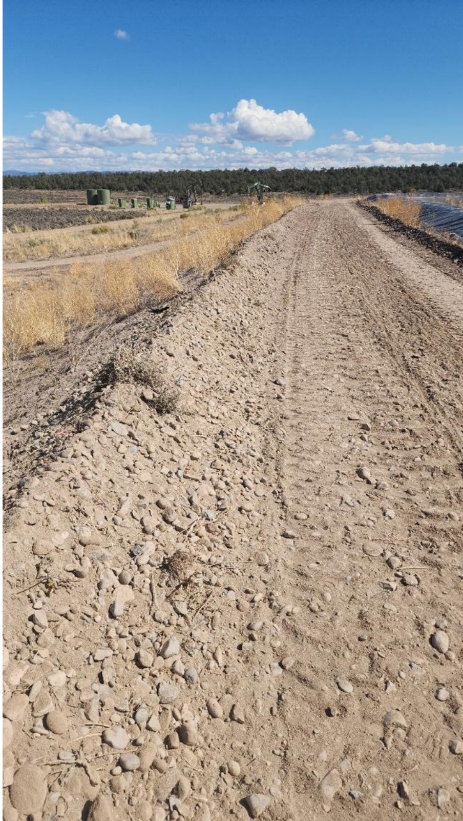
Photo 6: September 26, 2025. Repaired erosion along access road, north side of TUA. Post Repair.
