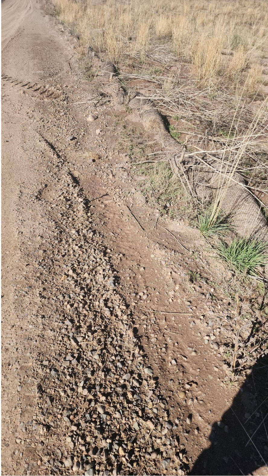
Photo 13: October 17, 2025. Straw Wattles displaced by significant precipitation event. Pre Repair.
