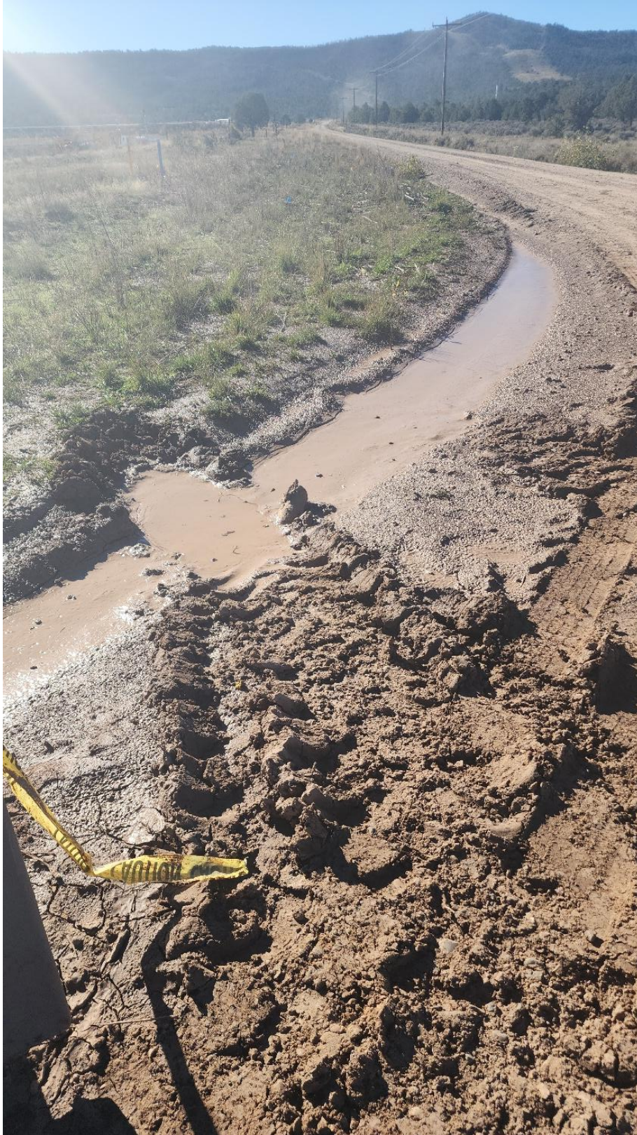
Photo 9: October 17, 2025. Well pad access road, significant precipitation event. Pre Repair.
