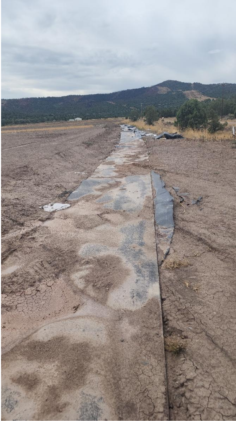
Photo 3: August 29, 2025. Un-bermed liner with sandbags along west side of TUA. Pre Repair.
