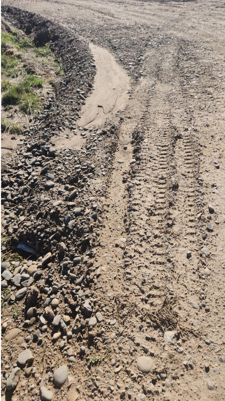
Photo 7: October 17, 2025. Culvert impacted by significant precipitation event, south well pad access road. Pre Repair.
