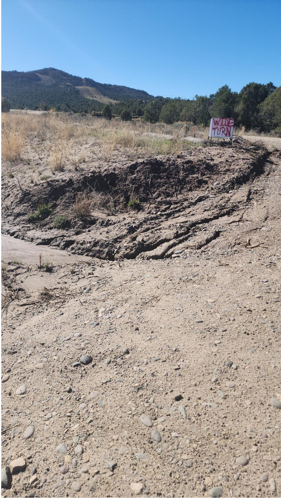
Photo 11: October 17, 2025. Erosional rills on TUA access road. Pre Repair.
