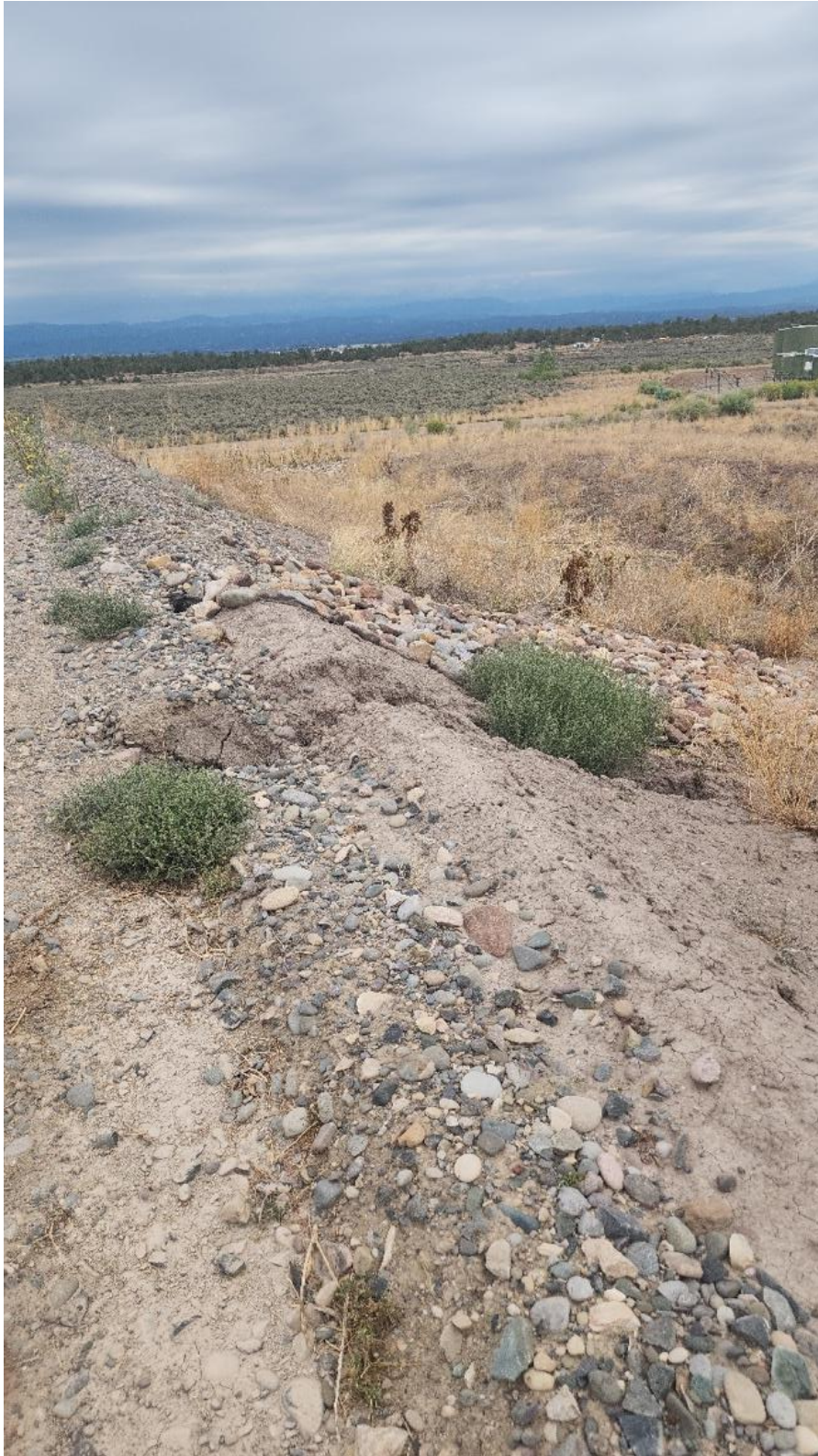
Photo 1: June 12, 2025. Erosion along access road, west side of TUA. Pre Repair.
