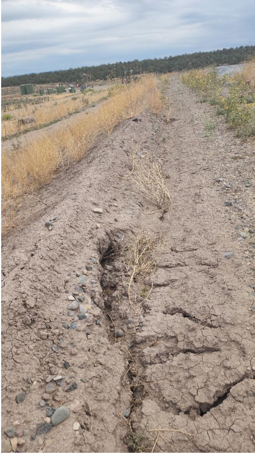
Photo 5: August 29, 2025. Erosion along access road, north side of TUA. Pre Repairs.
