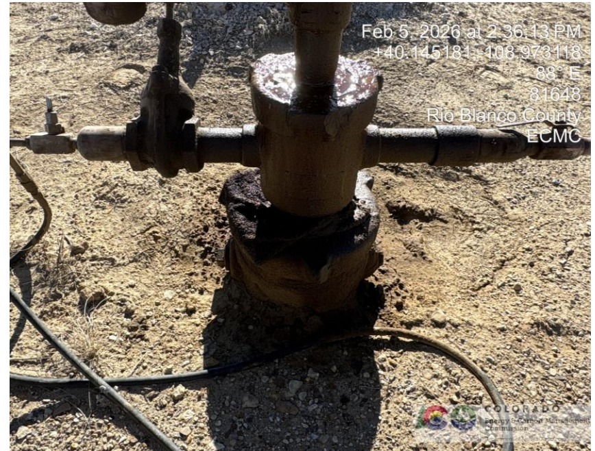
Photo # 1749 Bradenhead inaccessible
