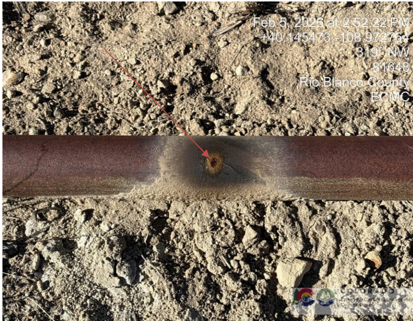
Photo # 1776 Possible flowline lacks integrity
