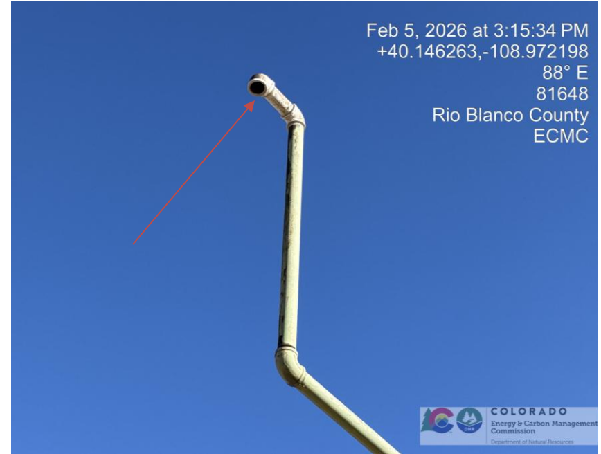
Photo # 1813 Open ended piping/wildlife hazard/available for entry by wildlife
