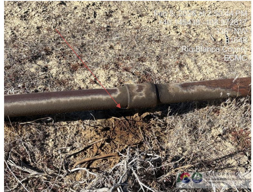
Photo # 1774 Staining/Weeds/undesirable plant species presents a potential fire hazard
