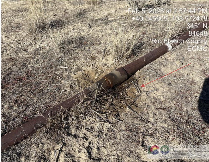
Photo # 1784 Staining/Weeds/undesirable plant species presents a potential fire hazard
