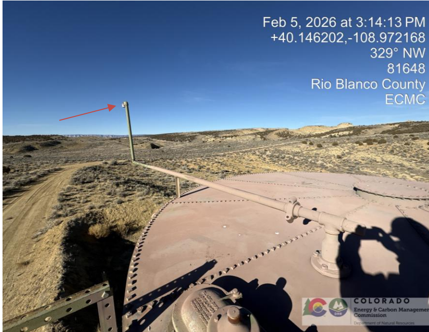
Photo # 1810 Open ended piping/wildlife hazard/available for entry by wildlife
