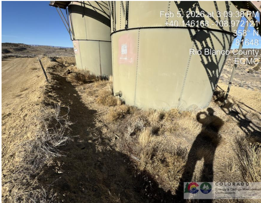
Photo # 1799 Weeds/undesirable plant species presents a potential fire hazard
