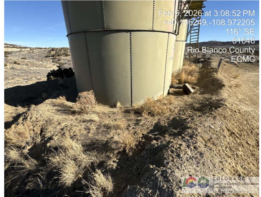
Photo # 1798 Weeds/undesirable plant species presents a potential fire hazard
