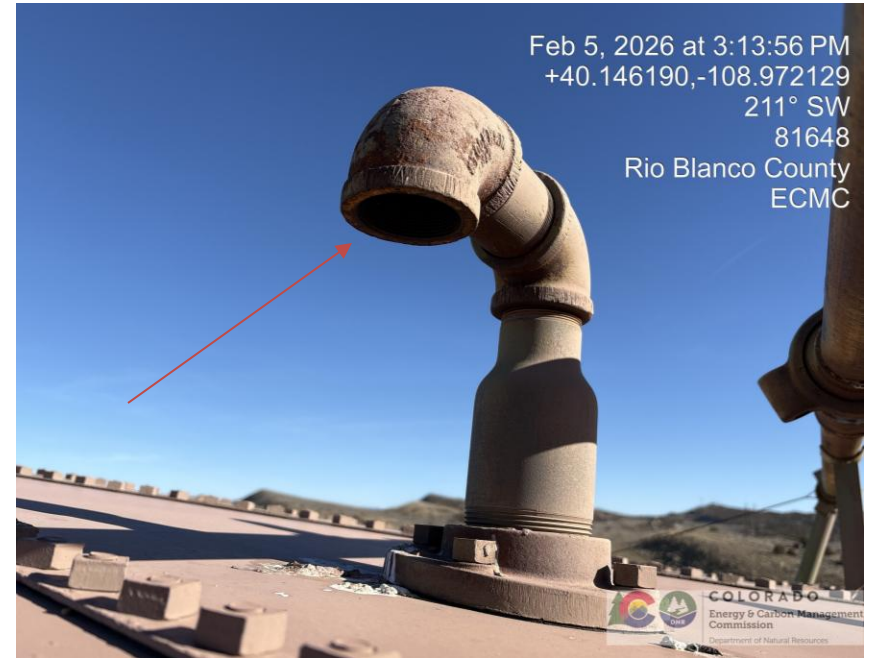
Photo # 1808 Open ended piping/wildlife hazard/available for entry by wildlife
