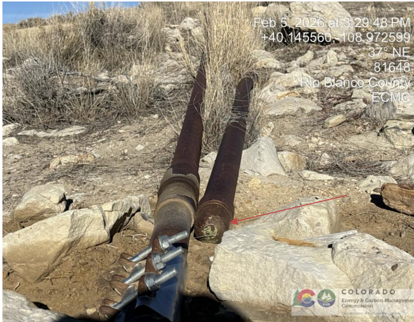
Photo # 1829 Unused flowline lacks lockout tagout (OOSLAT)
