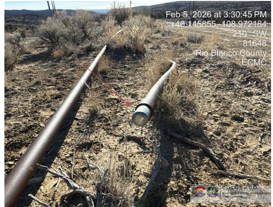
Photo # 1830 Unused flowline lacks lockout tagout (OOSLAT)
