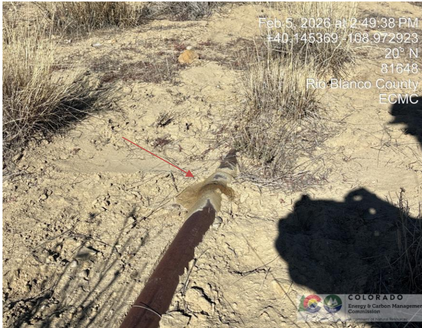
Photo # 1772 Staining/Weeds/undesirable plant species presents a potential fire hazard
