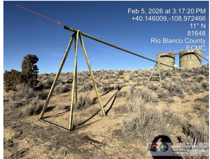
Photo # 1816 Unused unload line near tank battery not necessary for use on location
