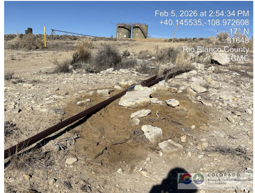
Photo # 1779 Staining/Weeds/undesirable plant species presents a potential fire hazard
