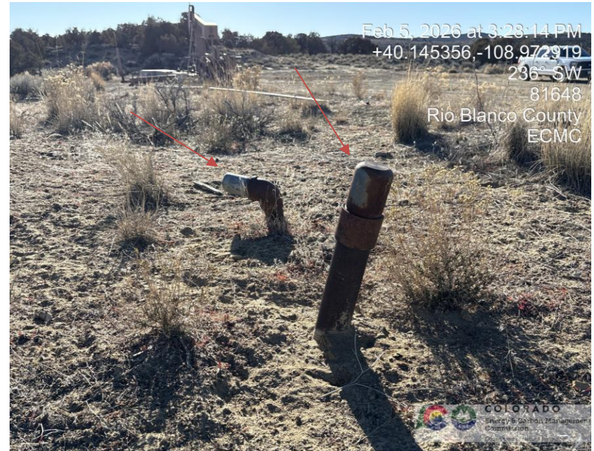
Photo # 1827 Unused flowlines lack lockout tagout (OOSLAT)
