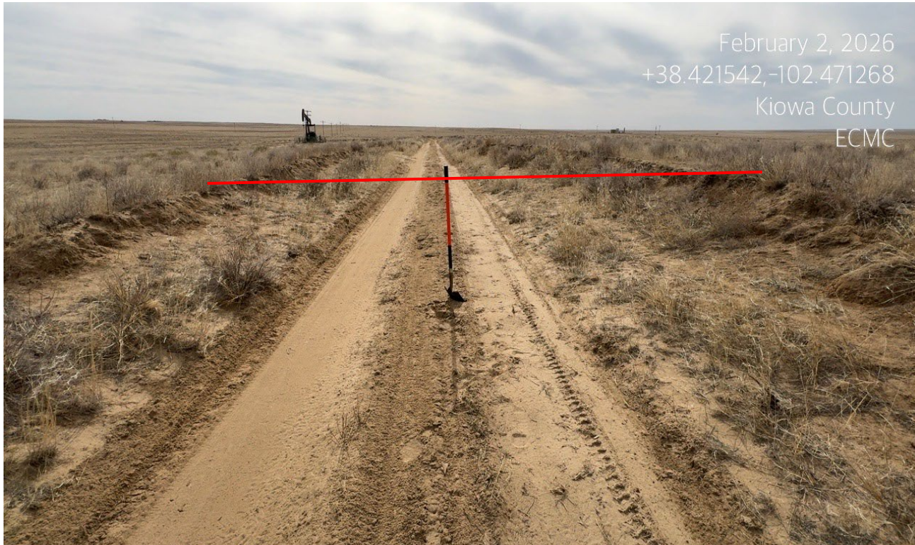
Photo 2. Facing south along the main access road. Overtime, the road has wind eroded causing a swale in the road. Red arrow is the approximate original grade and the shovel is 4.5 feet for scale.
