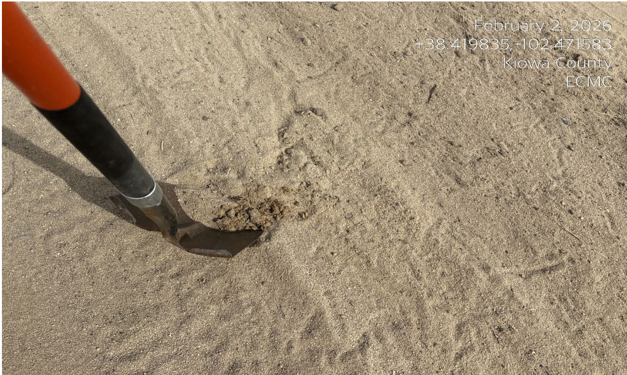
Photo 7. The road consists of loose sandy soil which is susceptible to further erosion.
