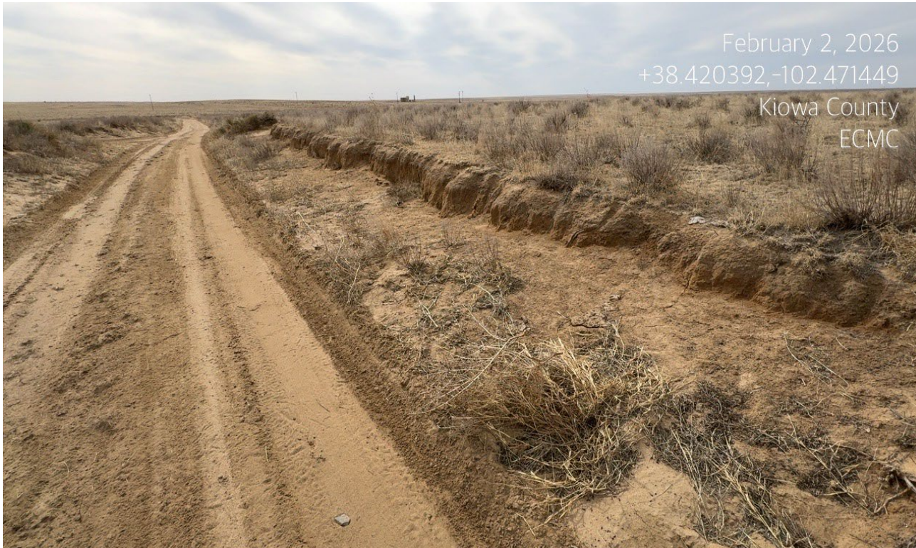
Photo 3. The road side near the location is not stabilized and is eroded.
