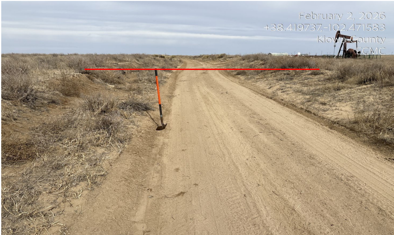
Photo 6. Facing north along the main access road. Overtime, the road has wind eroded causing a swale in the road. Red arrow is the approximate original grade and the shovel is 4.5 feet for scale. The well site is in the upper right of photo.
