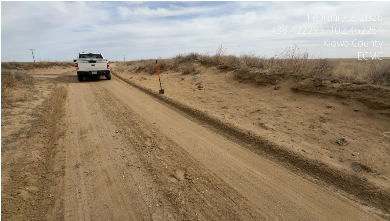
Photo 3. The roadside has eroded and is not stabilized with vegetation. The sandy soils are susceptible to further erosion. This area needs to be repaired and stabilized.
