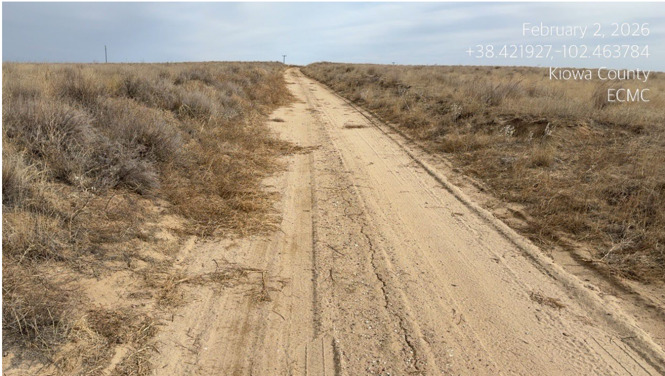
Photo 1. Facing east along the main road. The road is swaled and below the original grade of the terrain. There is concern for winter snow to blow onto the road impeding vehicle passage.
