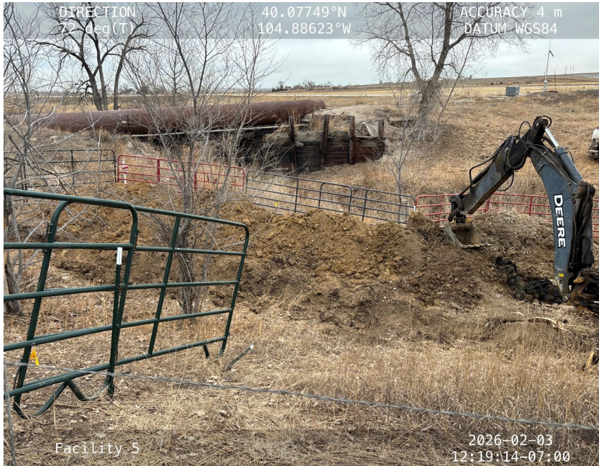
Impacted oily stockpile
