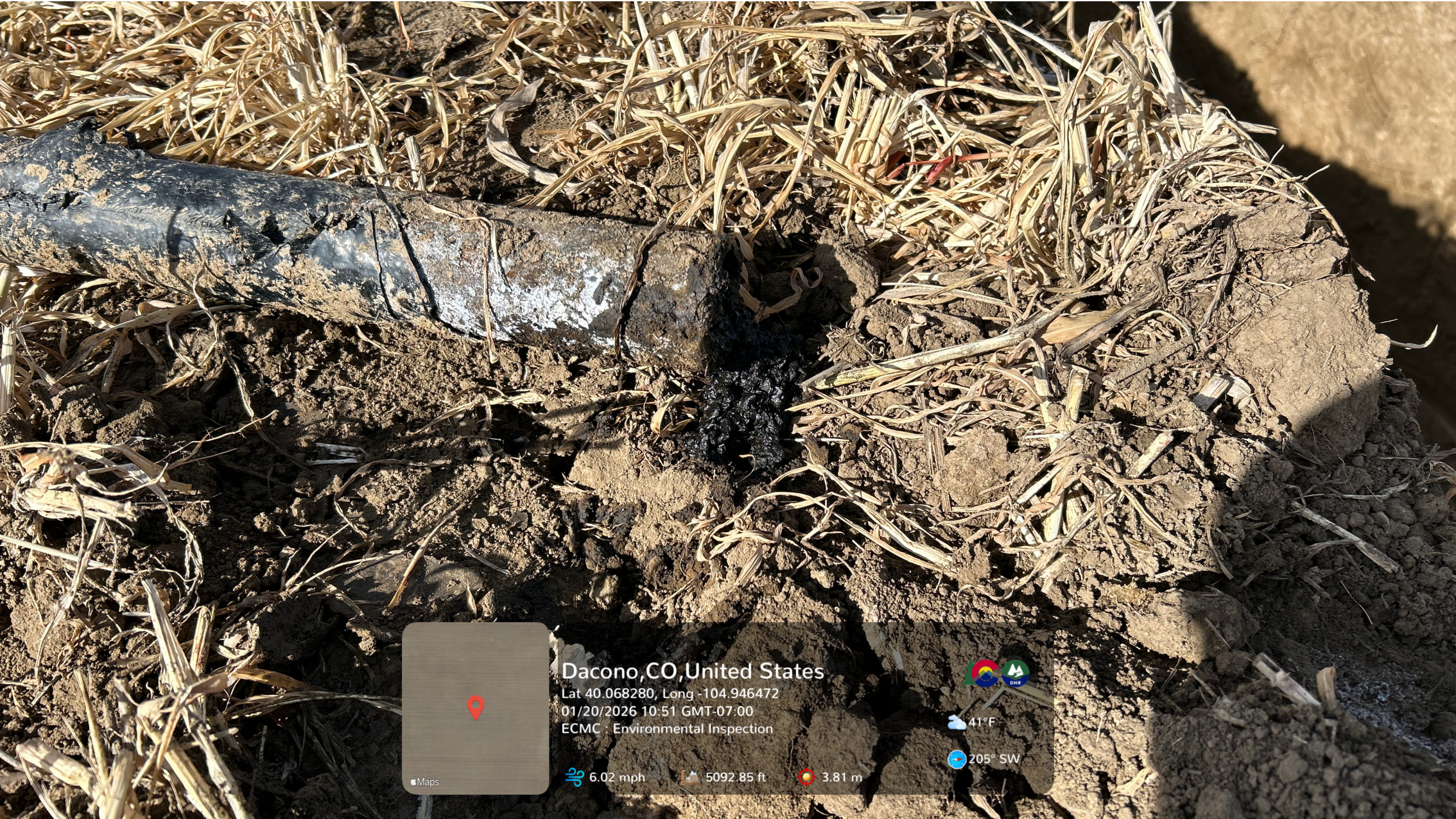
(Closer view of flowline from previous photo). Petroleum hydrocarbon residue is visible on the ground surface at the end of the removed segment of flowline.
