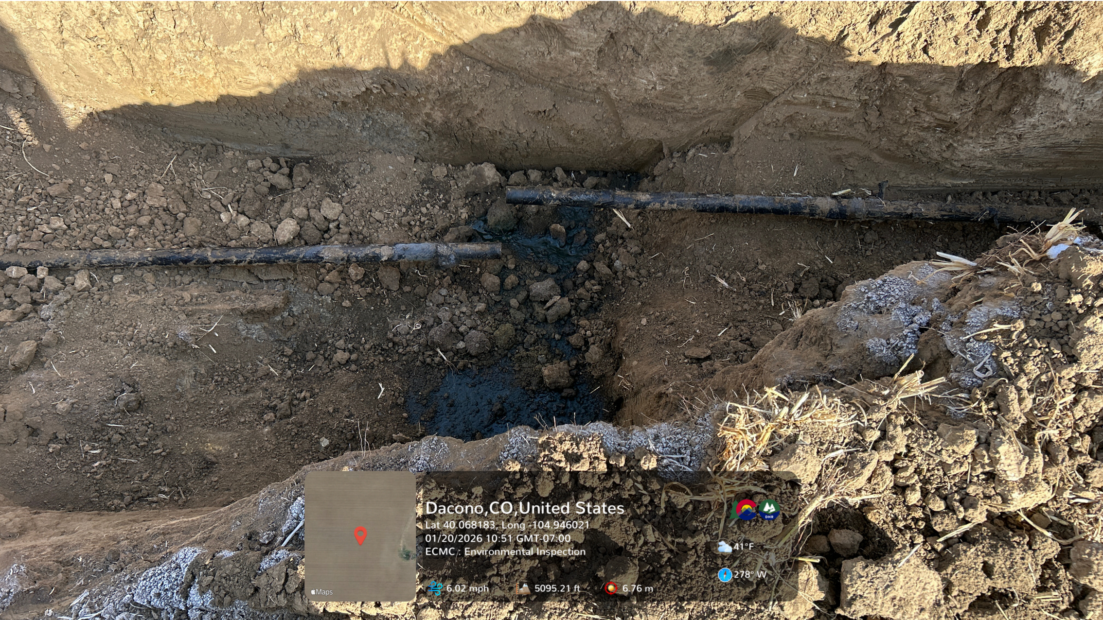
Looking at a second area of impacts to soil. Pooled petroleum hydrocarbon fluid is visible under a cut segment of flowline.
