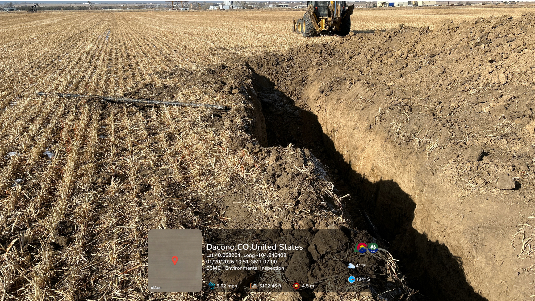
Looking at the western endpoint of the trench. A segment of flowline has been removed and placed on the ground surface adjacent to the trench. (Zoomed in on next photo).
