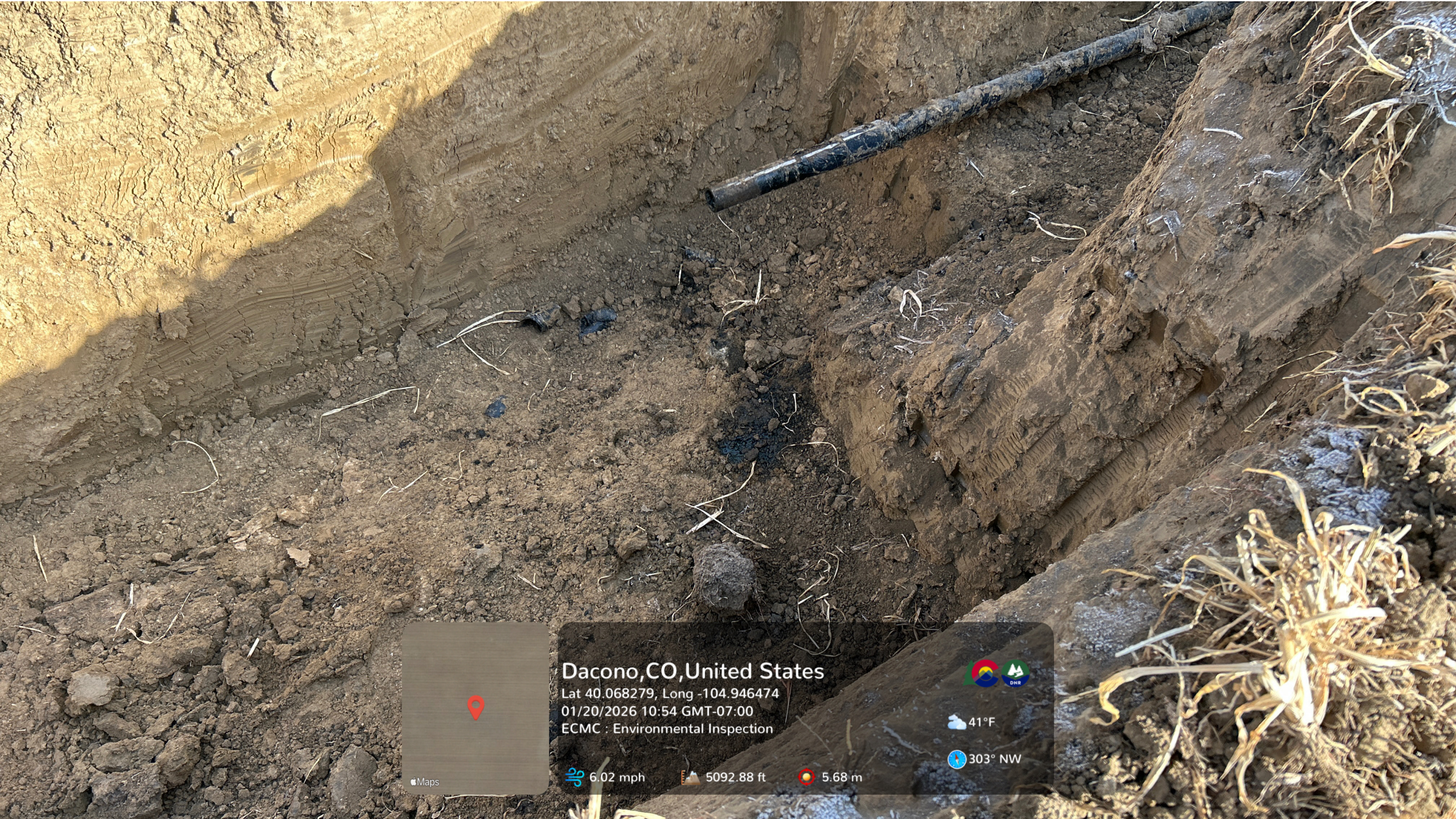
Looking at a third area of impacts to soil. Pooled petroleum hydrocarbon fluid is visible under a cut segment of flowline.
