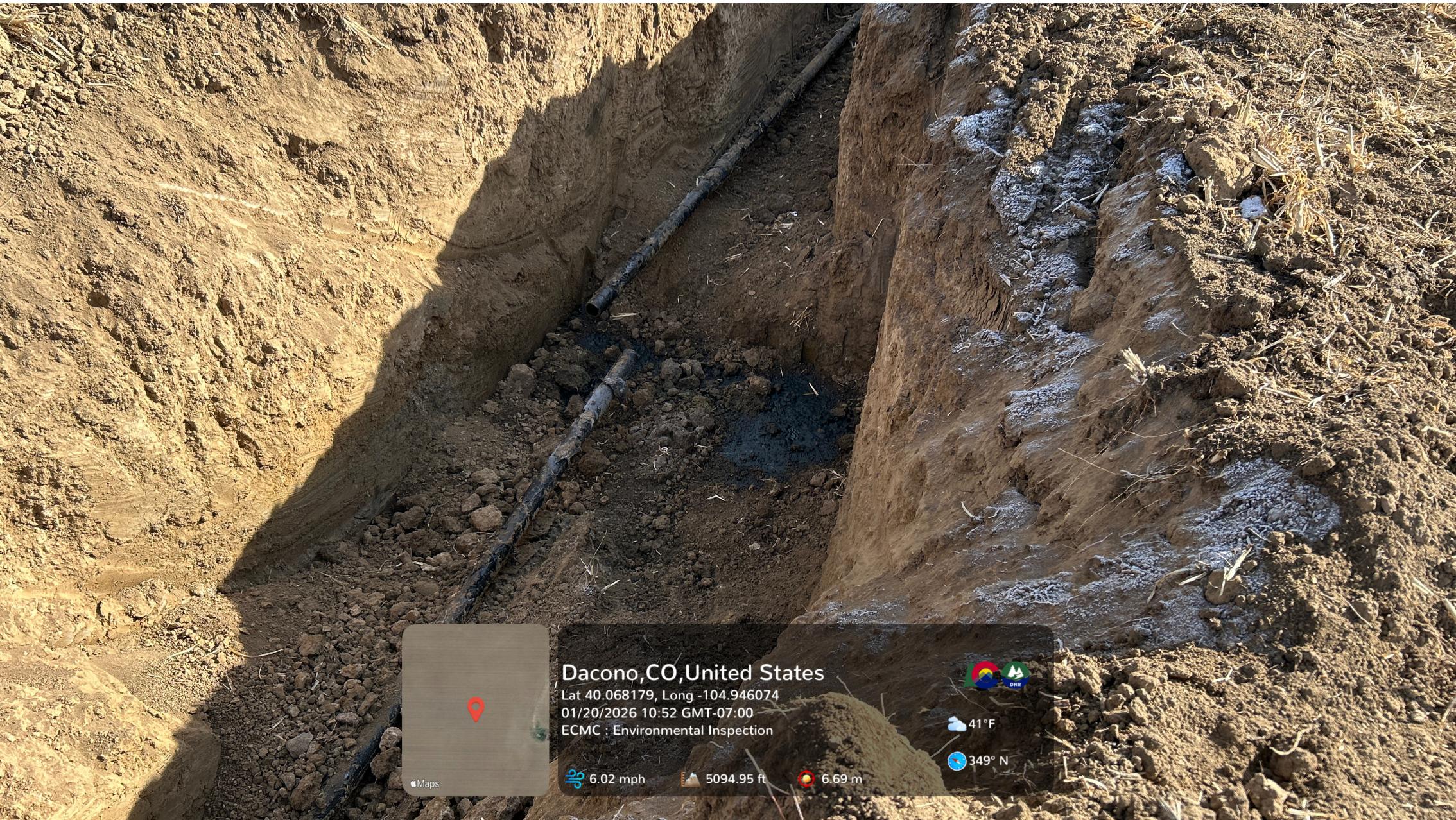
Looking at the second area of impacts to soil. Pooled petroleum hydrocarbon fluid is visible under a cut segment of flowline.
