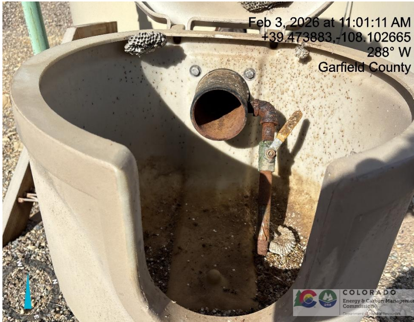
Photo # 8035 Open ended load line
