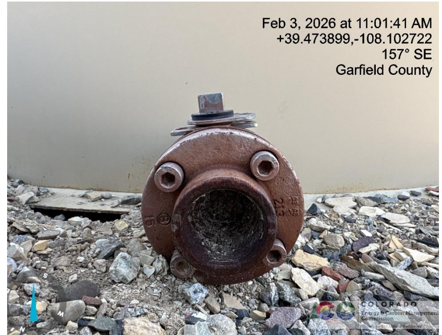
Photo # 8036 Open ended load line
