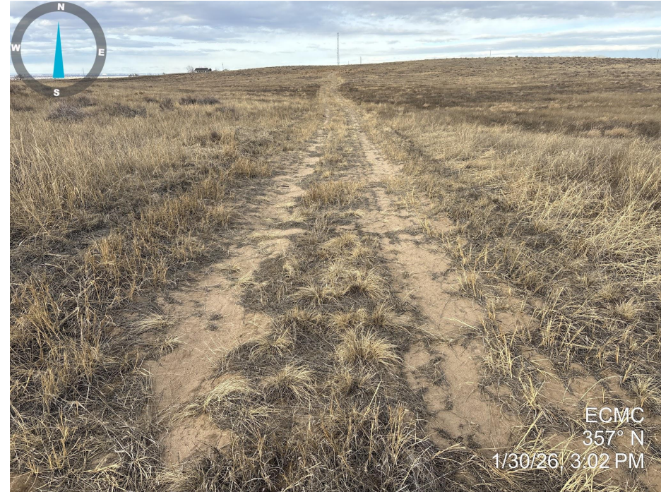
Photo 6. Photo taken of the access road to the location. Photo illustrates that final reclamation does not meet Rule 1004 standards along the road as bare ground remains.
