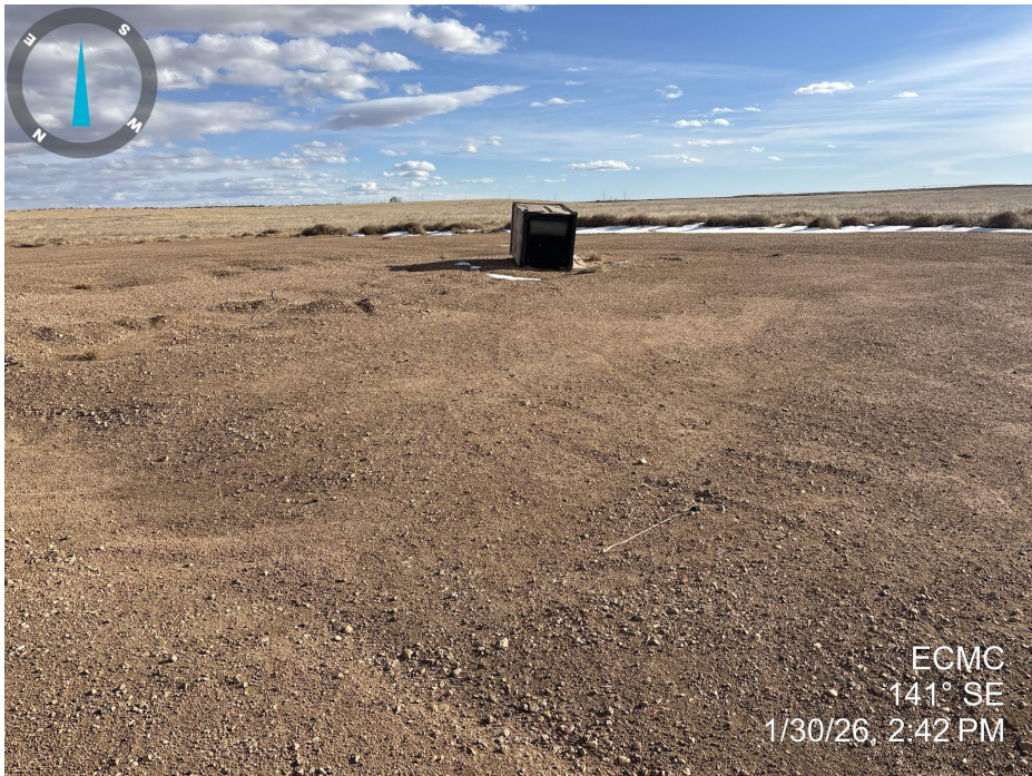
Photo 9. Photo taken of the tank battery location, facing southeast. See comments under Photo 8.
