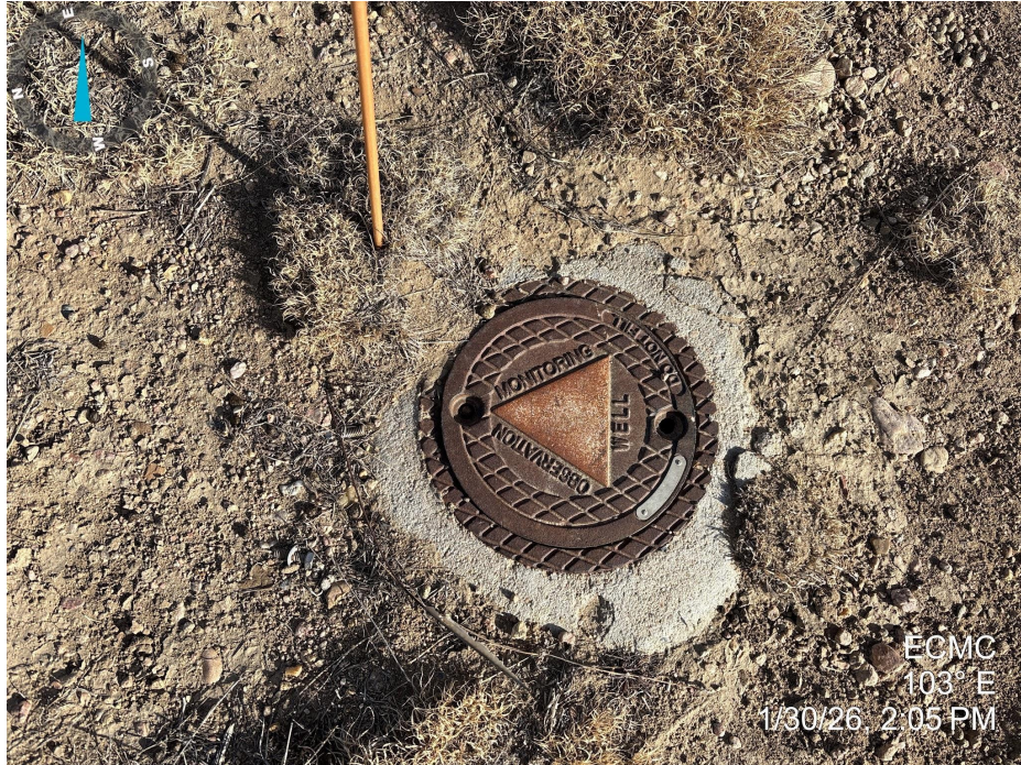
Photo 5. Photo taken of an observation monitoring well at the location.
