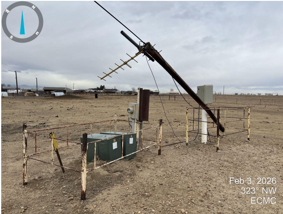
Photo 3. Photo taken at the transformers and control station to the west of the pumpjack. A signal pole is broken off and wedged in the fencing.
