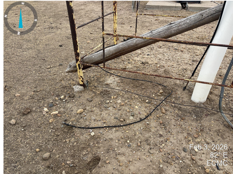
Photo 4. The signal pole cable is disconnected.
