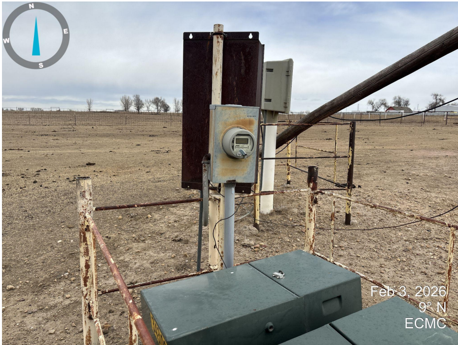
Photo 5. Meter has power.
