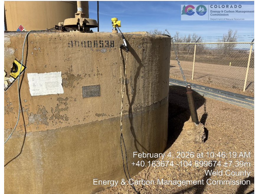
Produced water tank and anchors
