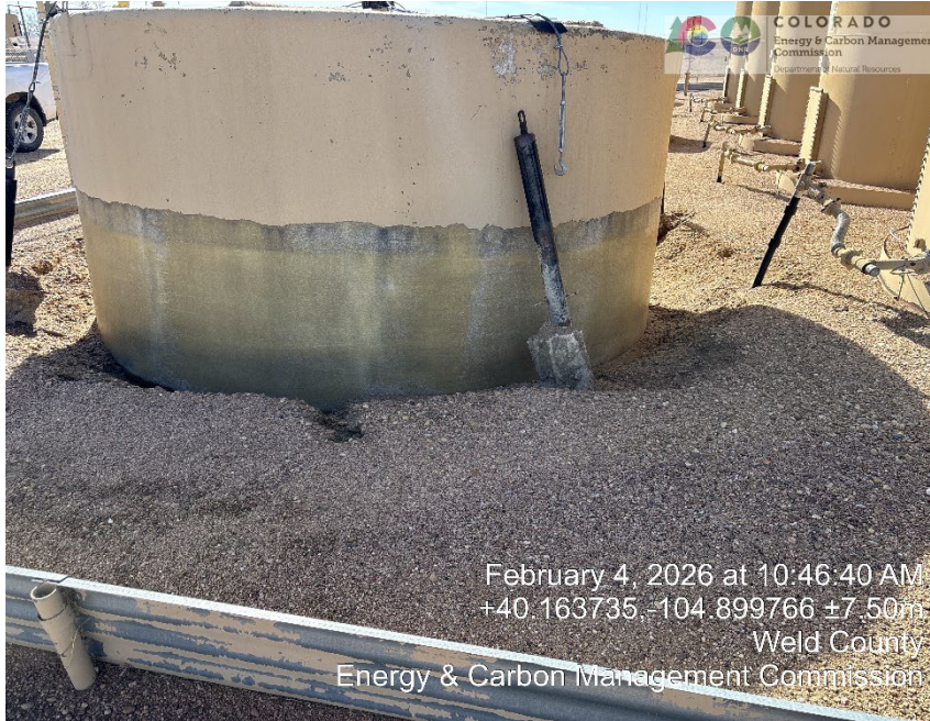
Produced water tank and anchors
