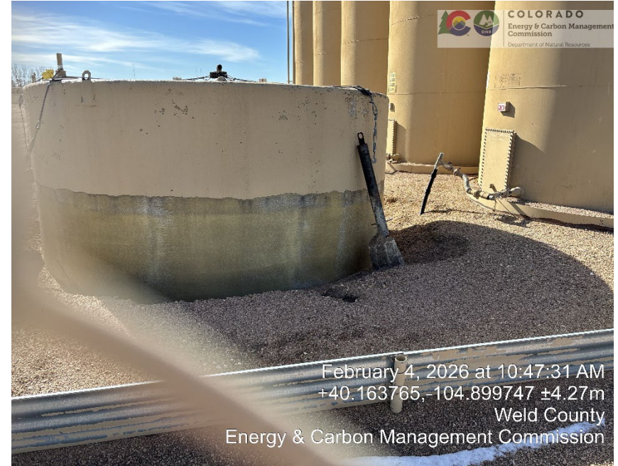
Produced water tank and anchors
