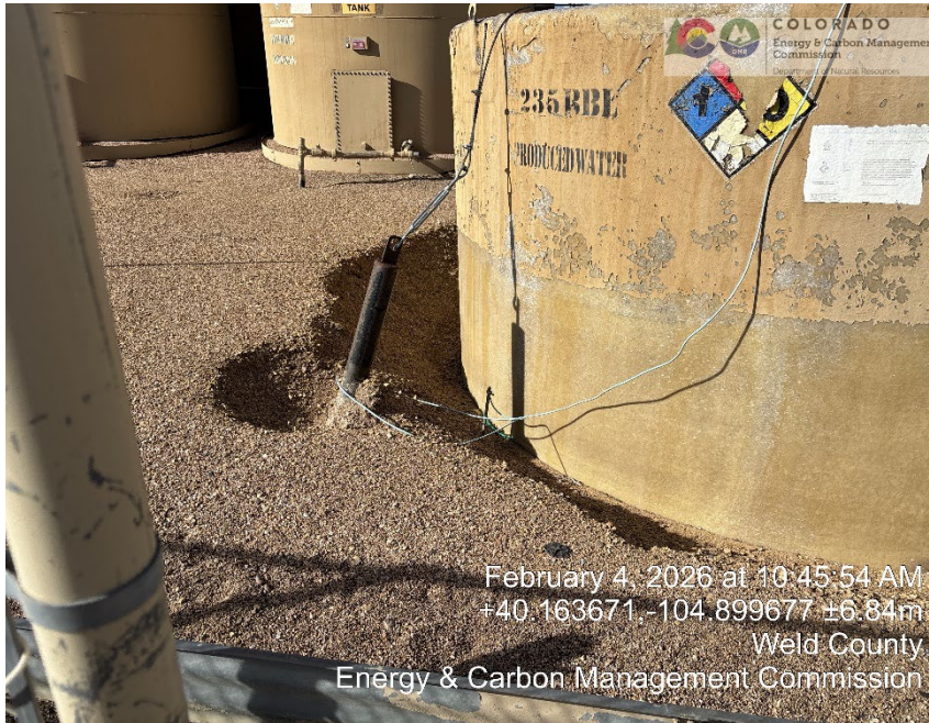
Produced water tank and anchors
